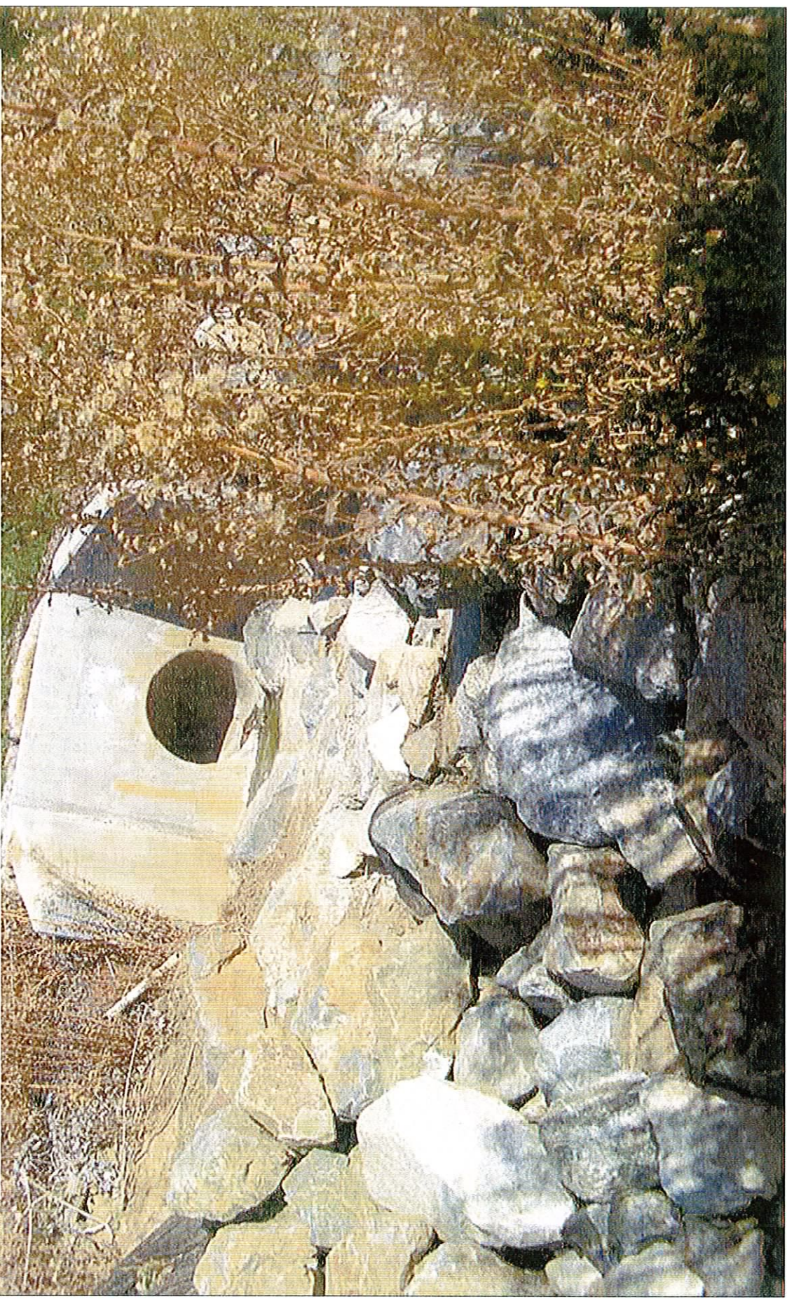
Outfall headwall from sediment basin with rip rap for Phases 1-5 (The Plateau)
