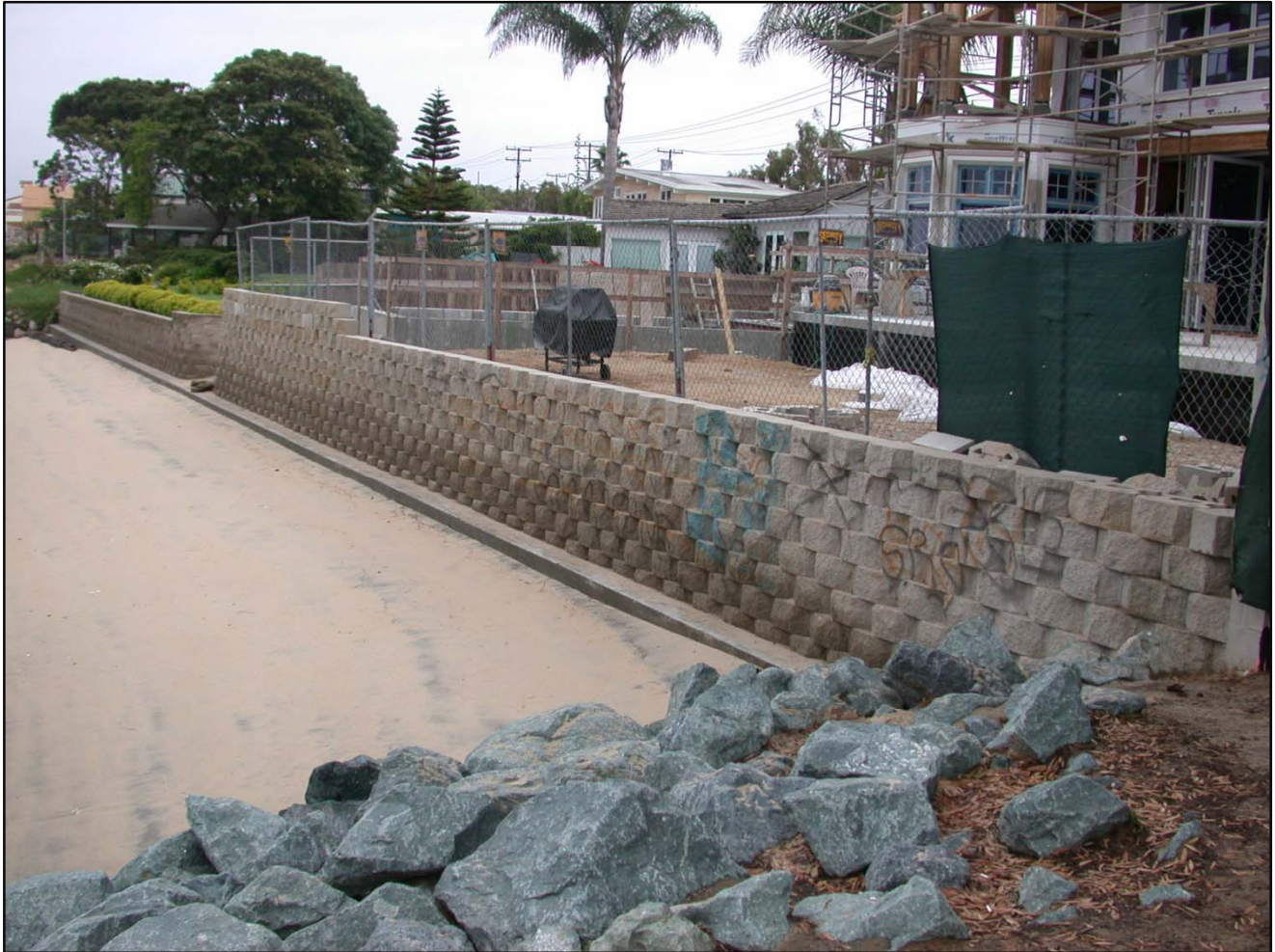
Figure 2. Seawall and exposed beach at 501 and 505 1 st street, May 9, 2008.
