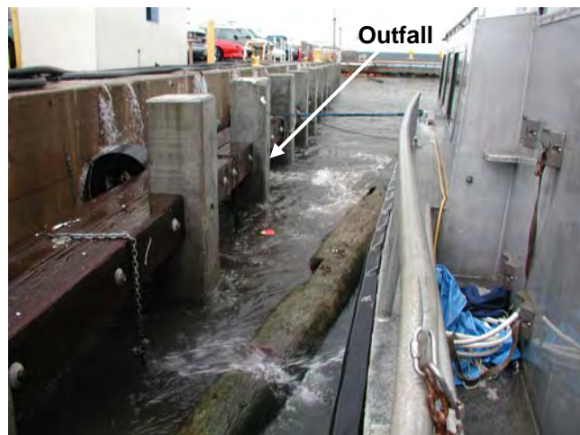
Fig. 3. RV ECOS tied up along quay wall outside OF14. The sensors and pump intake were directly in line with the outfall. Note sheet runoff over quay wall.
