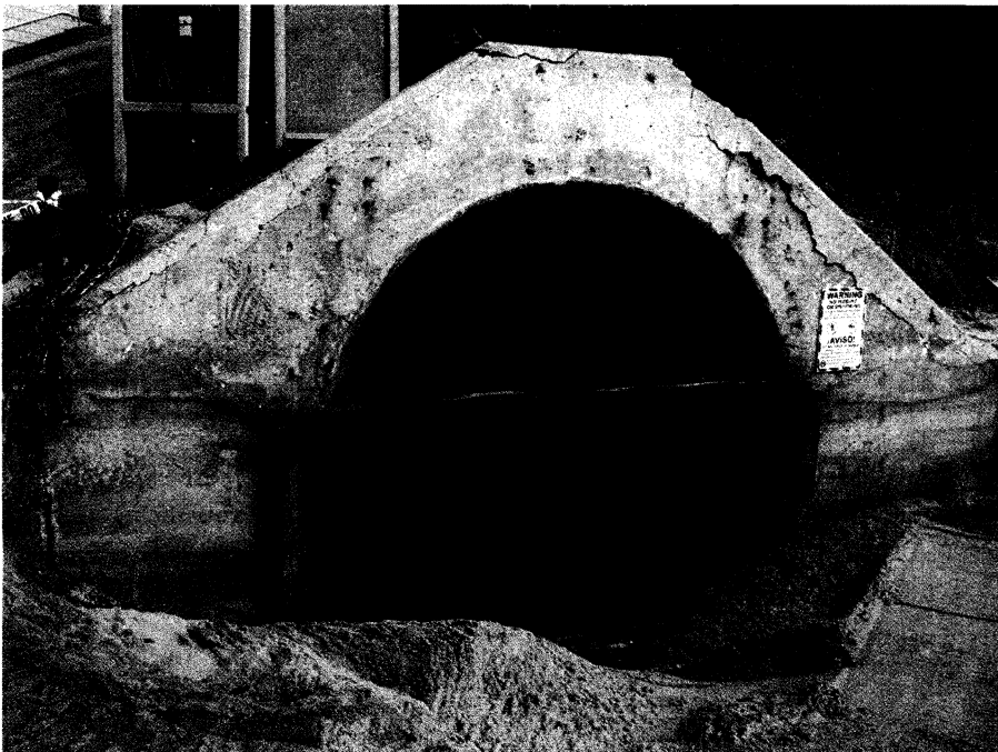
Figure 10 - The outlet to the storm drain is partially blocked by wood.
