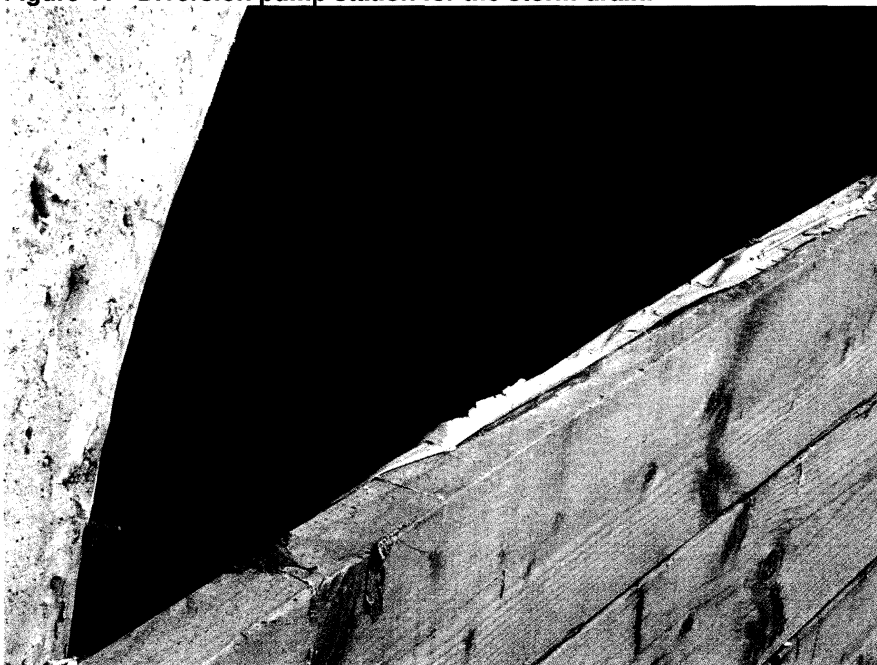
Figure 12 - Close up of the storm drain outlet and the blockage. There is still some water inside.
