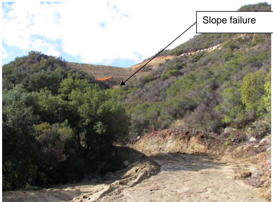
Figure 7. Photo of failed slope at 38175 Via Vista Grande. (IMG_060.JPG taken by San Diego Water Board on December 16, 2008.)
