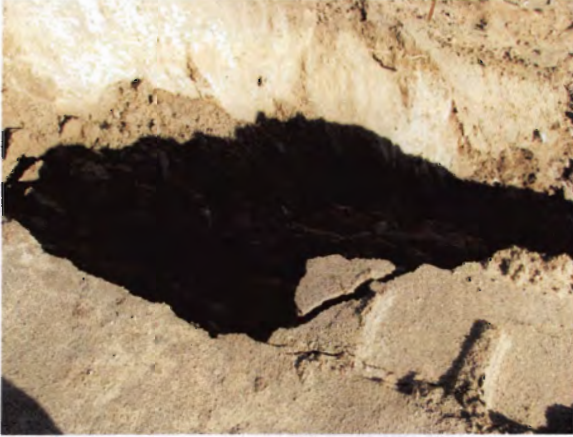
Photo 10: Failed slope along access road
