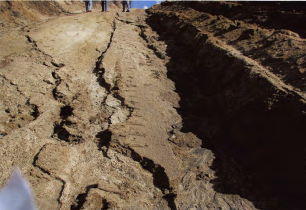
Photo 18: Road leading to basin is heavily eroded. The slopes along the roads are not stabilized to prevent erosion.
