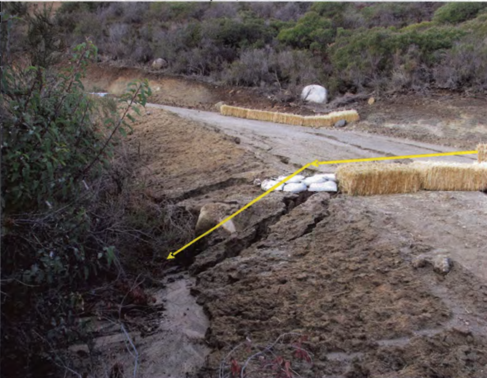
Photo 20: The road was constructed (w/o proper permit) directly across a natural waterway. Erosion effects can be seen across the road.
