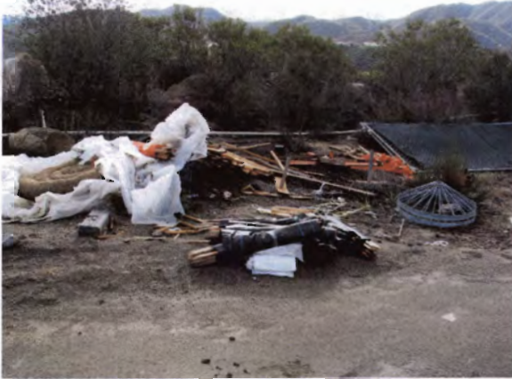
Photo 22: Construction wastes littered along fire-road
