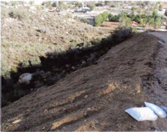
Photo 08: Outside slope not stabilized, discharge of fill (rocks, boulders, and vegetation) in waterway
