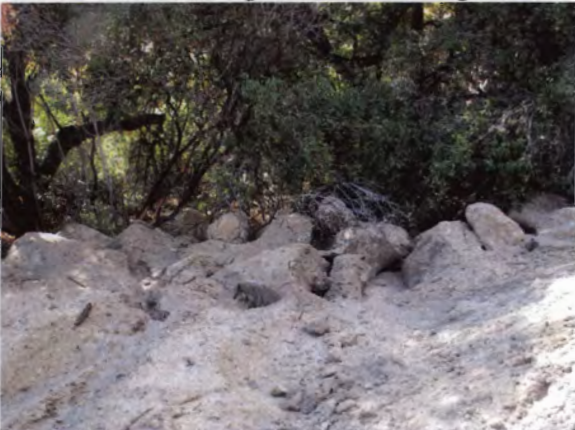
Photo 15: Sediment, silt and rocks are sidescaped into riparian corridor just downgradient from middle sediment basin
