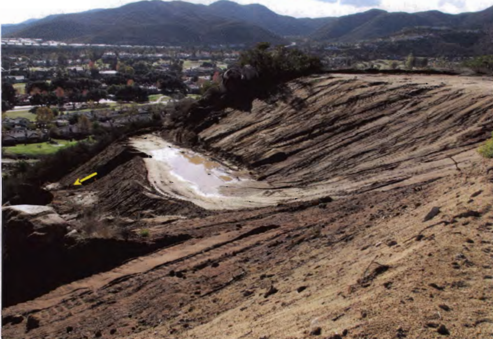
Photo 12: Failed sediment basin is unable to capture sediment-laden runoff from surrounding building pad.
