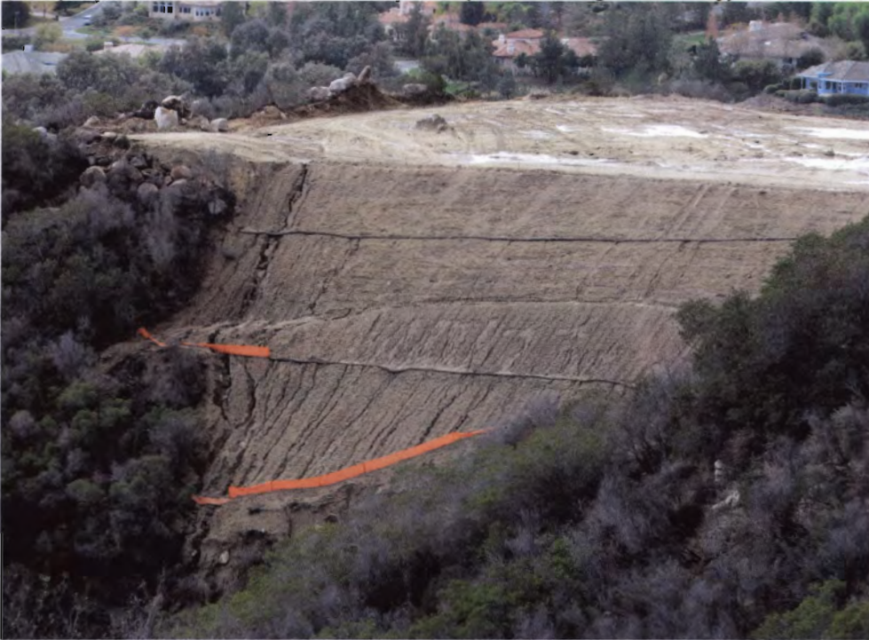
Photo 19: Failed BMPs on slopes; silt fence does not follow contour.
