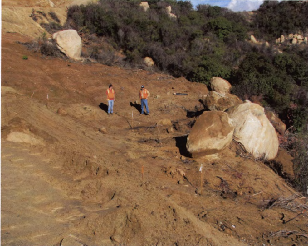
Photo 13: This area lacks erosion and sediment controls as significant quantities of dirt is placed alongside a natural waterway.
