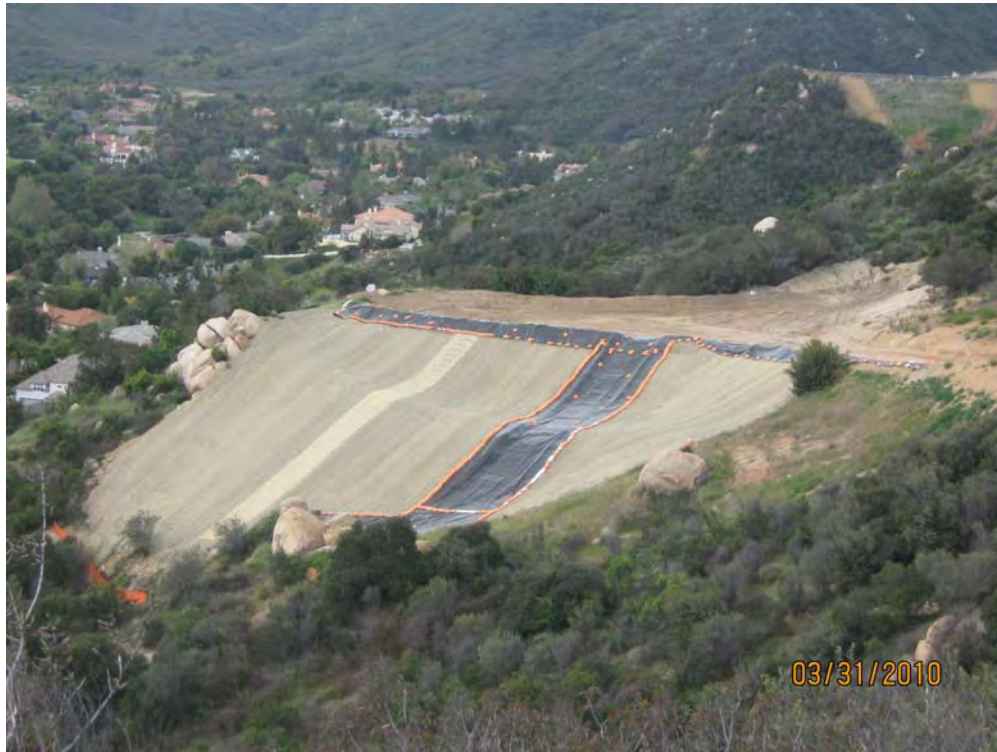
Figure 11. Photo of installation of proper erosion control at 38175 Via Vista Grande. (Photo IMG_040.JPG taken by County of Riverside on March 31, 2010.)
