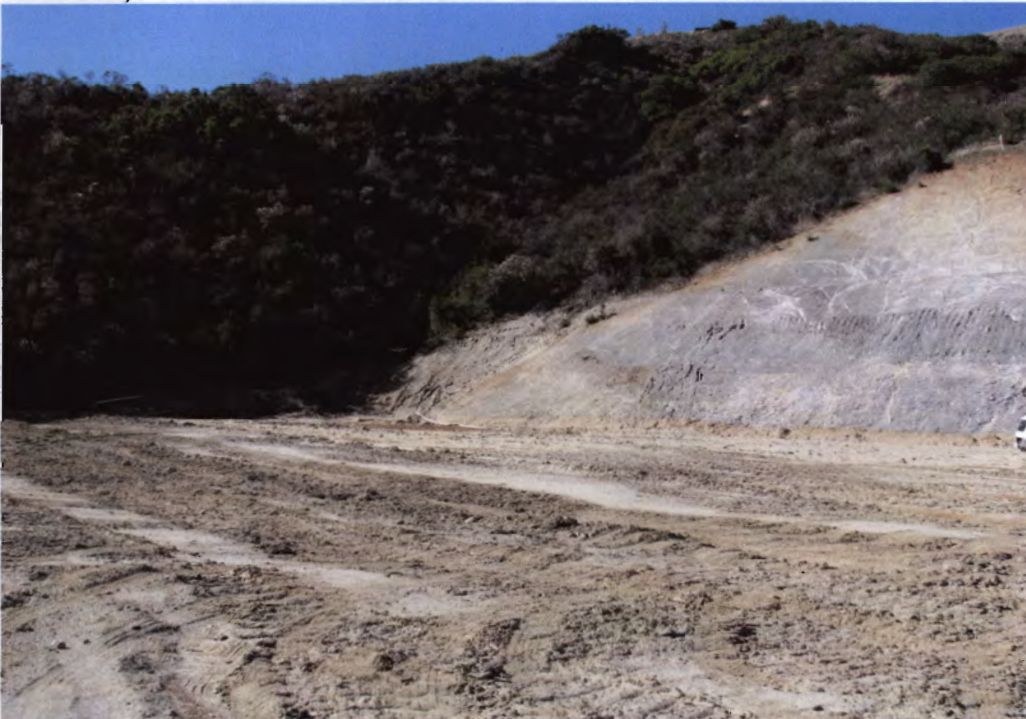
Photo 26: No slope stabilization and building pad is not covered or stabilized.
