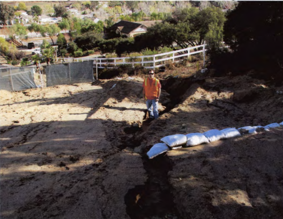
Photo 08: Erosion gullies were caused by high, concentrated storm water flows and failed BMPs.
