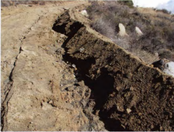
Photo 13: Shows severe erosion along access road leading to middle basin
