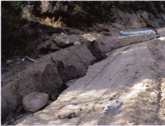
Photo 04: Erosion gullies along fire-road
