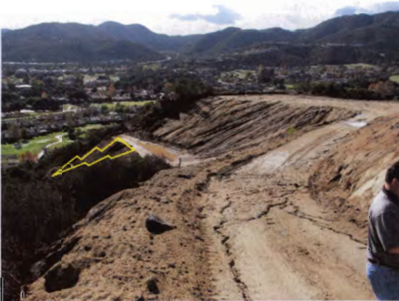
Photo 09: Unstabilized slopes and access road, breached sediment basin allowed sediment discharge (insert) in waterway
