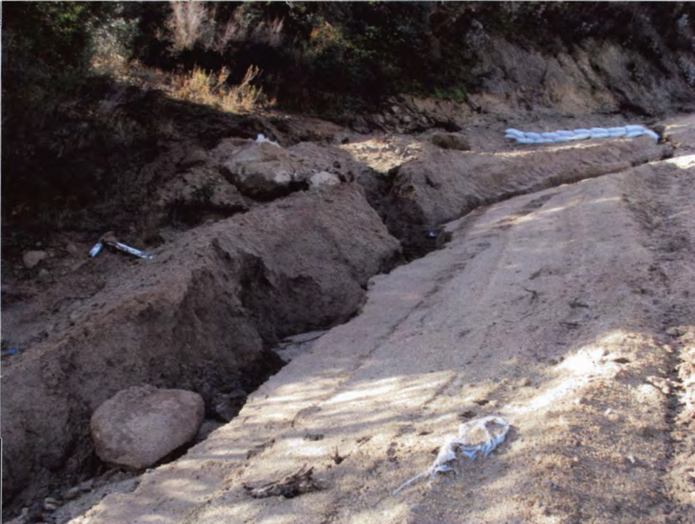
Photo 06: Erosion gullies along the fire road leading to Fairway Hills Estates site.
