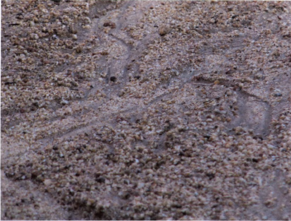
Photo 05: Close up of fire road shows extent of erosion-down to the bedrock
