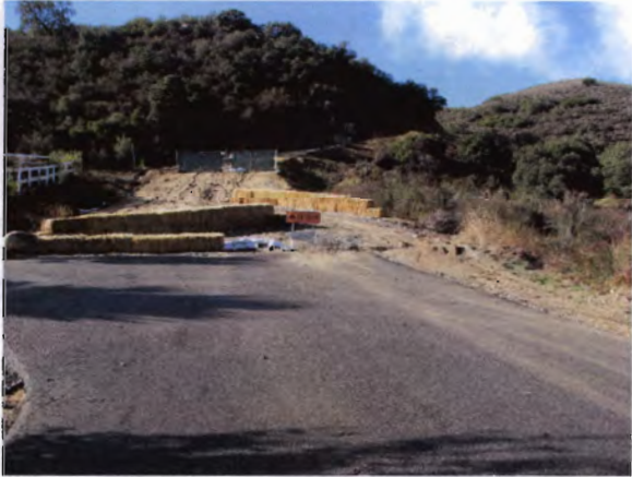
Photo 01: Site entrance at Claremont Street shows inadequate BMP to prevent erosion
