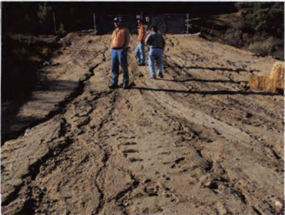
Photo 02: Shows fire-road with significant erosion at site entrance
