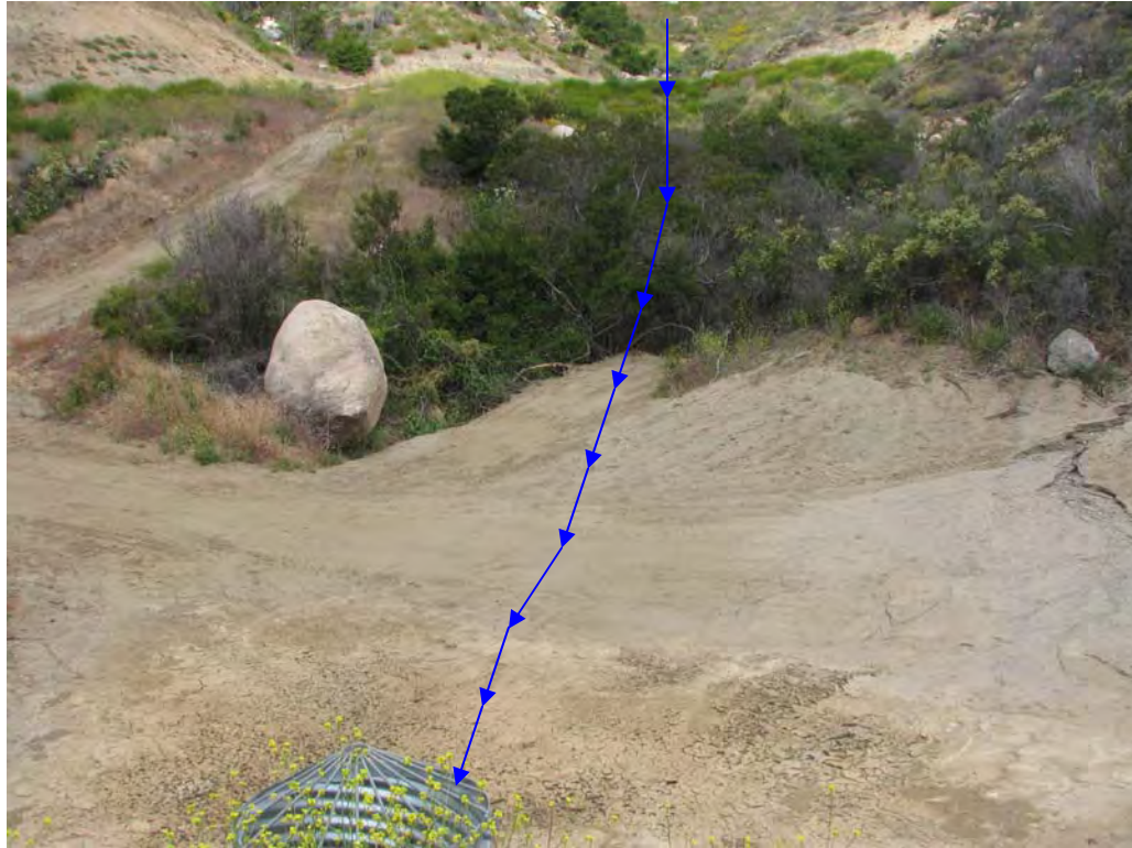
Figure 2. Photo from detention basin looking upstream. Blue arrow represents stream path. (IMP_0991.JPG taken by San Diego Water Board during May 11, 2010 inspection.)
