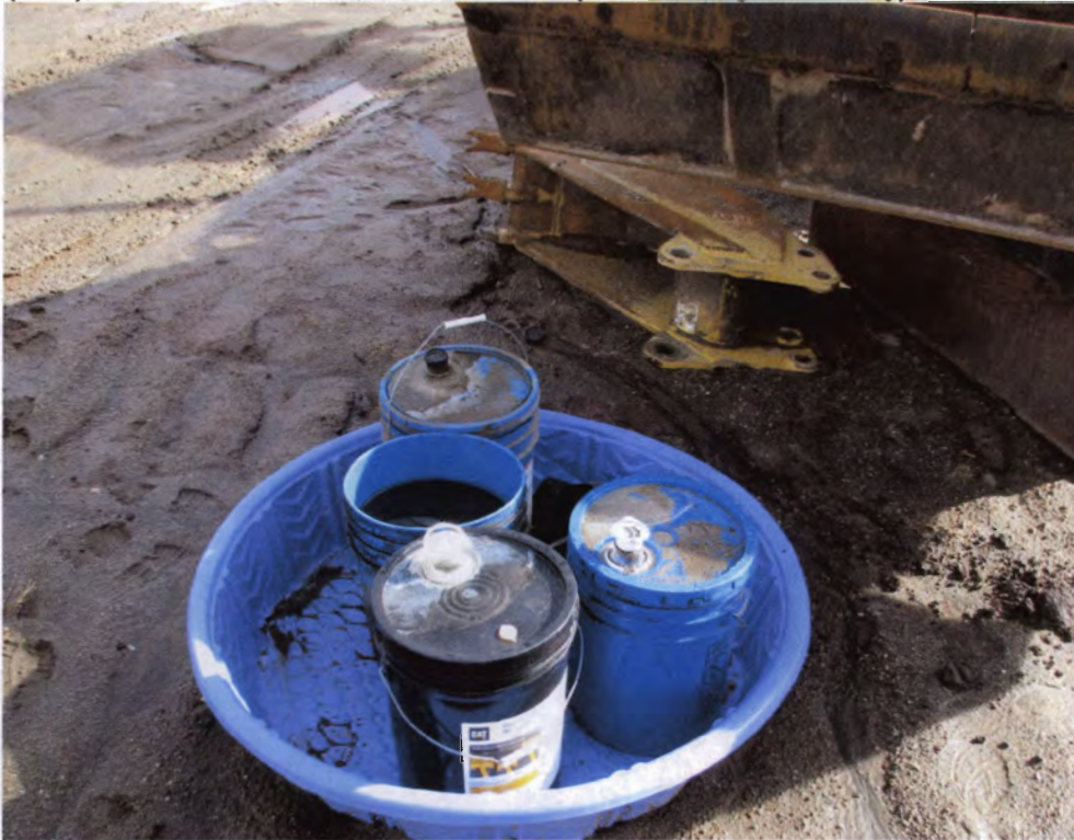
Photo 27: No BMPs to minimize exposure of mechanical construction wastes to stormwater or to potential accidents.
