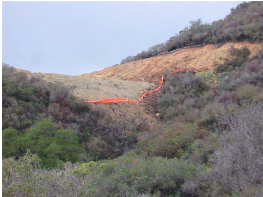
Figure 6. Photo of failed silt fence, and inadequately protected large graded slopes with numerous erosion rills. (Photo IMG_010.JPG taken by County of Riverside on January 29, 2008.)
