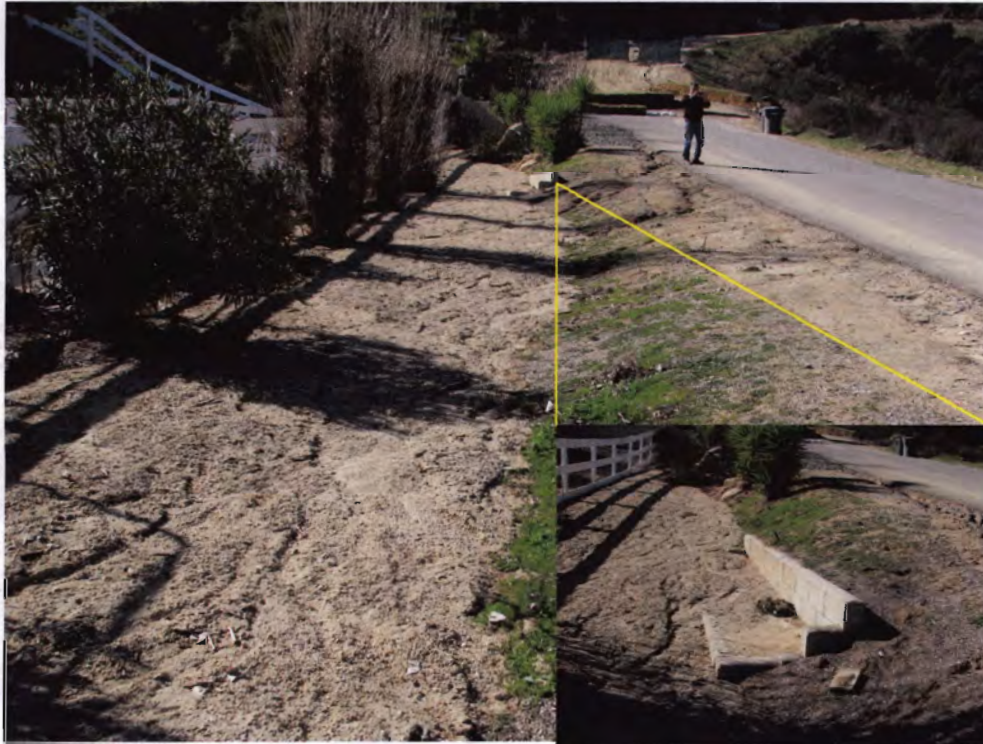
Photo 02: Sediment and silt are deposited along brow ditch along Claremont Street. Insert shows utility vault covered with sediment and silt.
