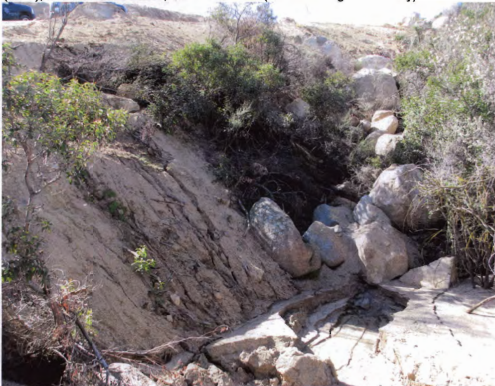
Photo 11: Rocks and boulders were sidescaped into the natural drainage area along the fire road. The caked sediment is evidence of flow blockage.
