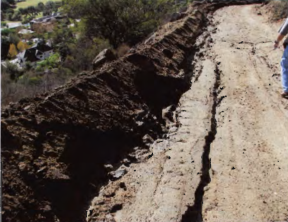
Photo 14: Looking downhill along access road shows erosion gullies
