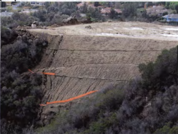
Photo 21: Close-up of erosion rills on slope shown in photo 20
