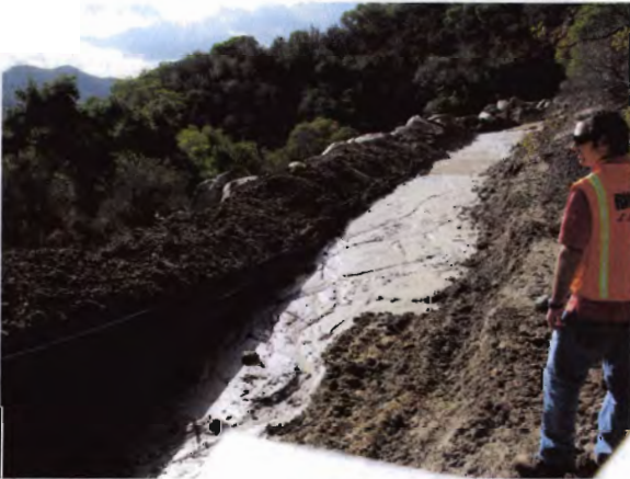
Photo 17: Shows significant sediment and silt in sediment basin
