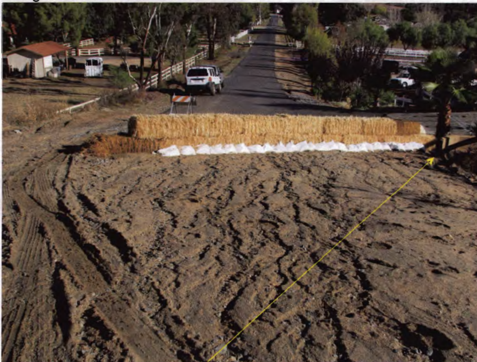
Photo 04: Looking east along Clairemont Street-site entrance/exit lacks tracking control. Insert shows point of sediment discharge under road crossing.
