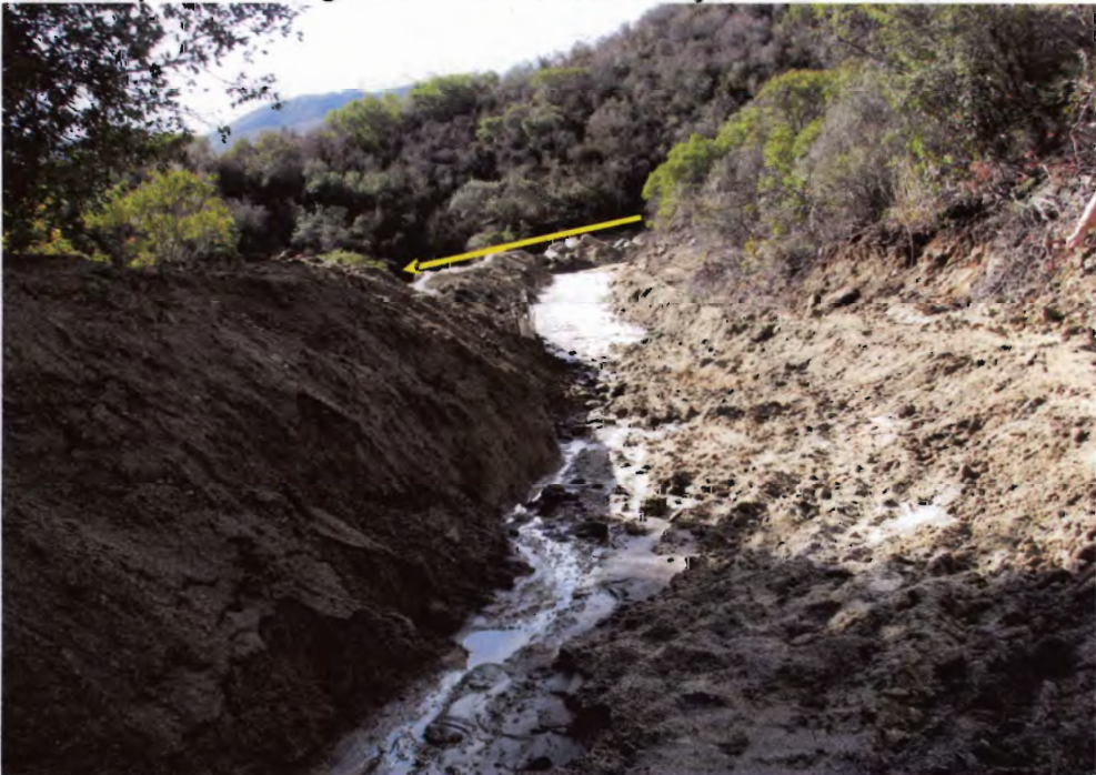
Photo 14: This sediment basin captures runoff from the fire road and upgradient construction activities. The basin is built directly in a natural waterway, shown in background.
