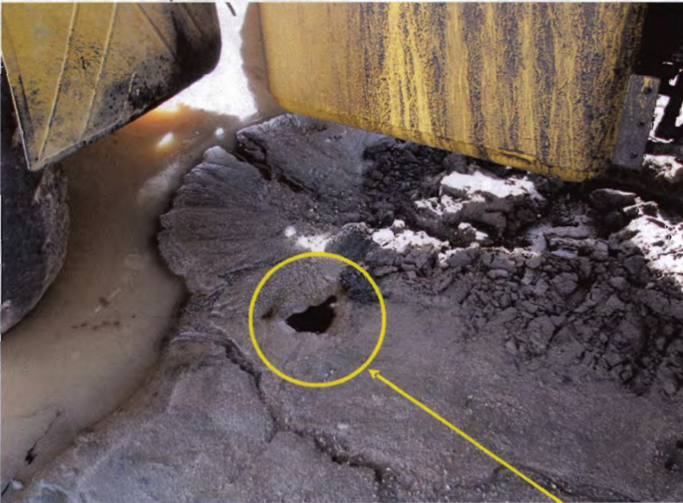
Photo 28: Construction vehicles are improperly stored with no drip pans to capture spill or leaks.
