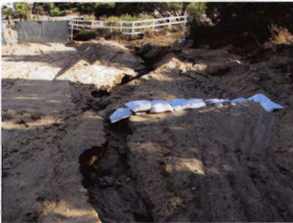
Photo 05: Erosion gullies leading to Claremont site entrance
