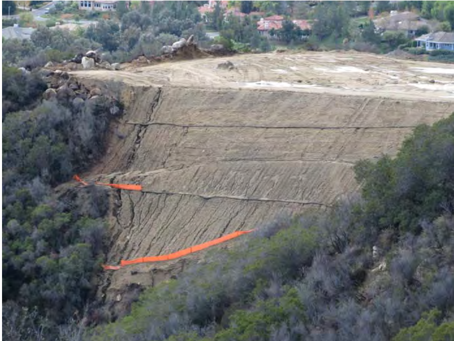
Figure 10. Photo of failed silt fences and erosion rills from 38175 Via Vista Grande. (IMG_077.JPG taken by San Diego Water Board on December 16, 2008.)
