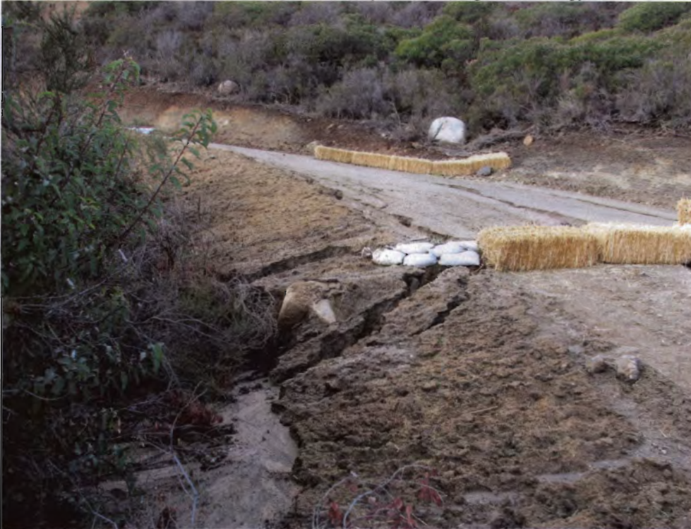
Photo 07: Inappropriate BMPs (hay bales and sand bags) are unable to contain and abate the high, concentrated flows causing rills and gullies.
