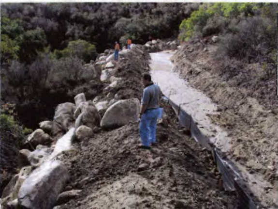
Photo 18: Construction wastes or fill (boulders, rocks, shrubs) sidescaped in waterway
