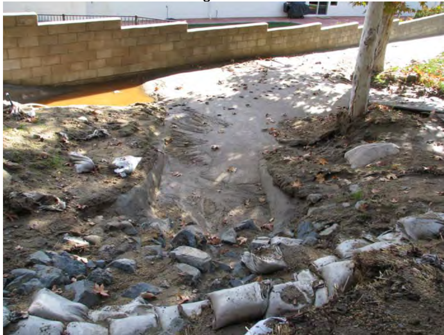
Figure 8. Photo of sediment discharge to MS4 tributary to Murrieta Creek.(IMG_0273.JPG taken by San Diego Water Board on December 23, 2008)
