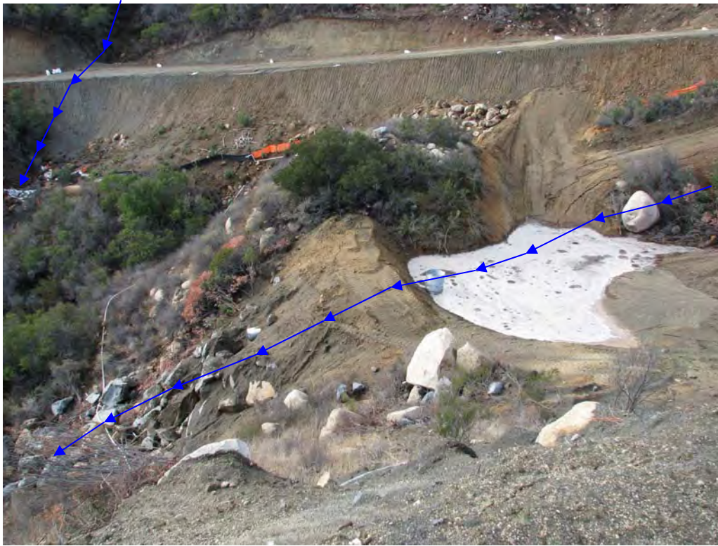
Figure 1. Photo of construction wastes/fill (sediment, silt, rocks, and boulders) discharged and detention basin construction in waters of the state. (IMG-081.JPG taken by San Diego Water Board during December 16, 2008 inspection.)
