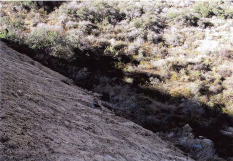
Photo 10: Evidence of recent grading of the fire road shows graded dirt was sidescaped down embankment towards natural waterway.
