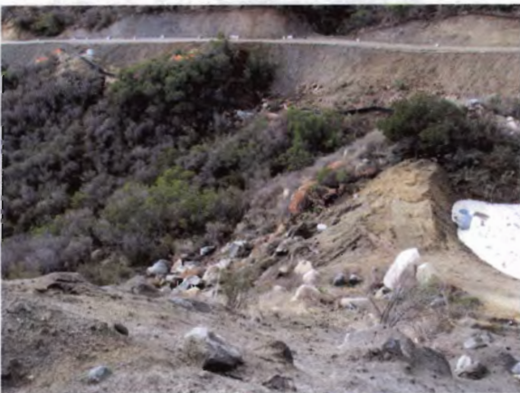
Photo 24: Construction wastes or fill (rocks, trash, and debris) deposited in waterway downgradient from the sediment basin. This sediment basin connects to the sediment basin shown in photos 17 and 18
