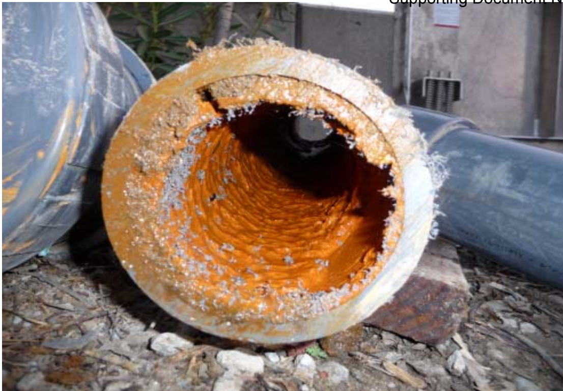
1. Fouling on Extracted Water Conveyance 1.
