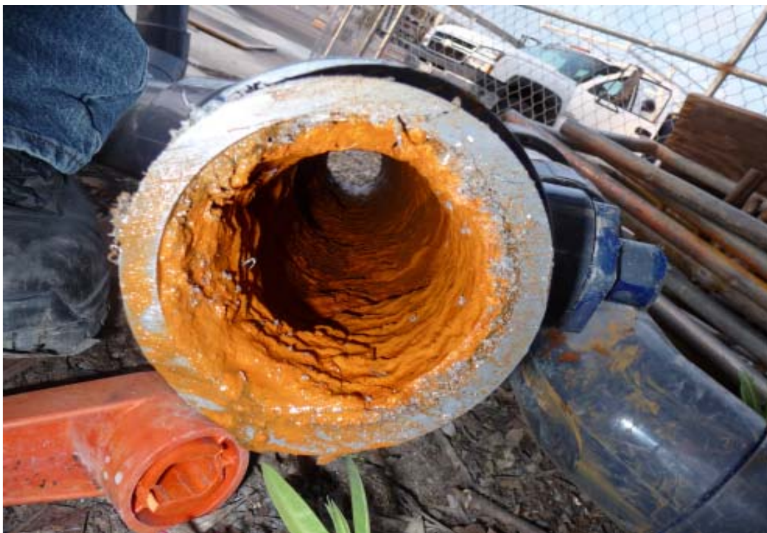
2. Fouling on Extracted Water Conveyance 2.
