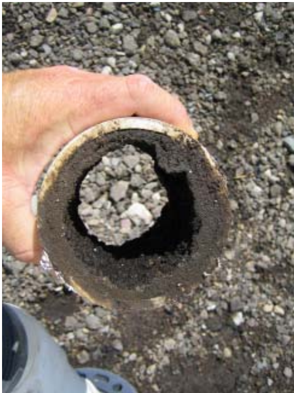
4. Mineral Fouling on Treated Discharge Pipe 2.
