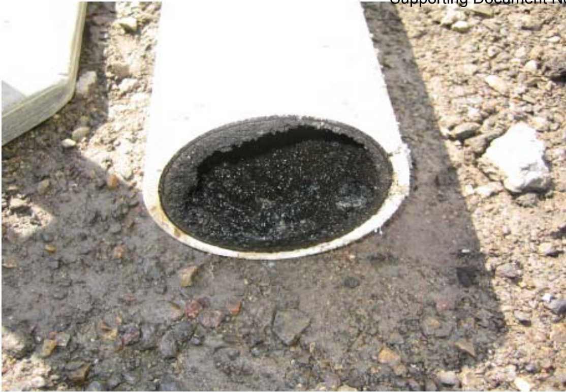
3. Mineral Fouling on Treated Discharge Pipe 1.
