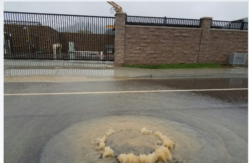
Harmony Grove Development Spill, Escondido, 02/17/17
