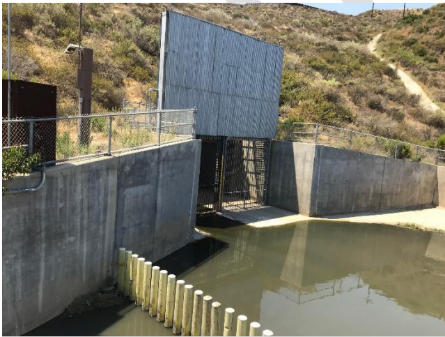
Ongoing wastewater pollution at Smuggler's Gulch canyon collector
