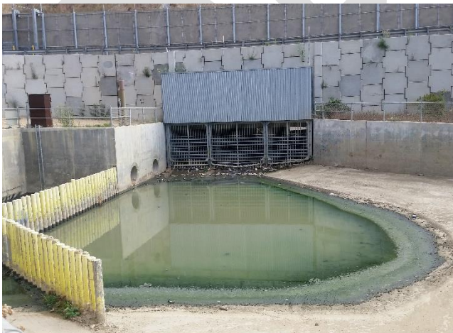
Wastewater pollution at Goat Canyon collector
