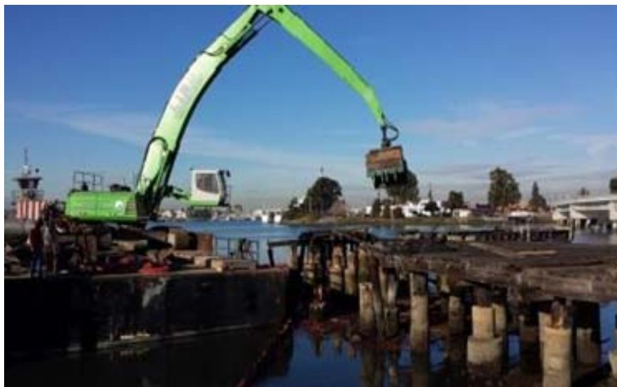
Photo 2b. Removal of the dilapidated pier at Union Point Park, Oakland, across from Coast Guard Island.
