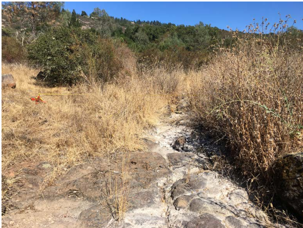
Photo 2: Upstream view through CH surveyed cross-section XS-1, approx. 100 ft. upstream of upper culverted road crossing. Tape line is visible mid-photo left.
