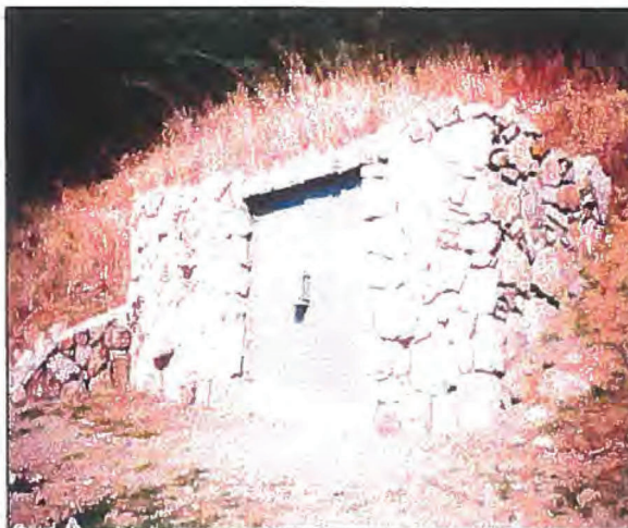
Figure 1-10. Bore Hole Enclosure at Spring No. 7
