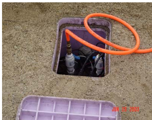
Photo 4. Surfactant injection ports
