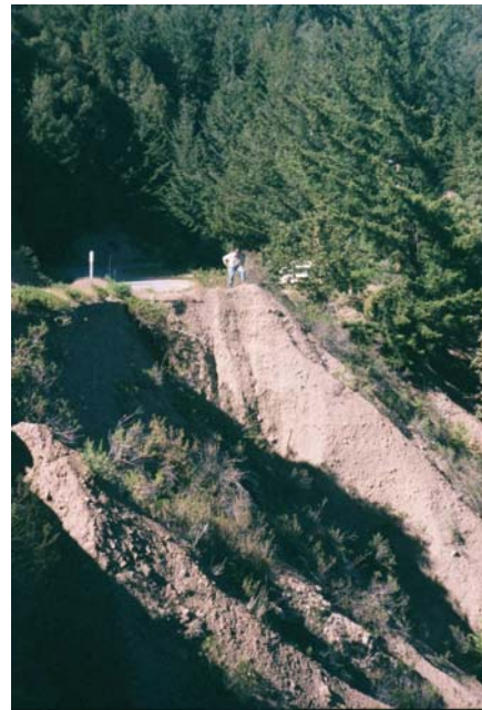
Figure 1. Landslide caused by a road
