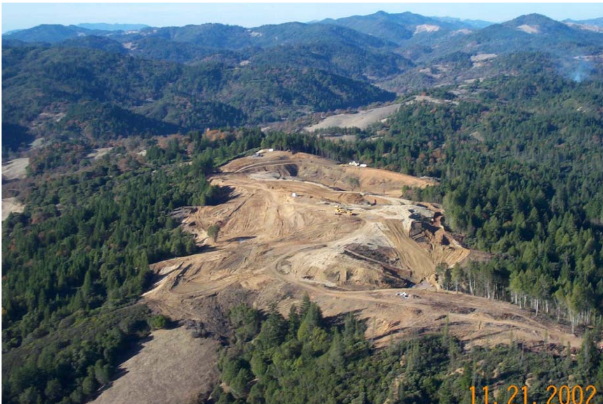
Eroding vineyard development located in the Eel River Watershed in Mendocino County, California. NCRWQCB fined the landowner $250,000 for sediment discharges that buried salmon spawning grounds.
