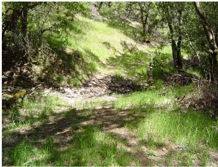
Figure 1. Trail Reconstruction – Some Erosion Problems Due to Heavy Rainfall in First Year.
