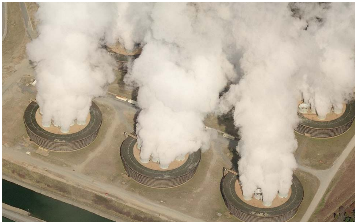
Figure 5-7 Bird's Eye View of Catawba's Non-Plume-Abated Mechanical Draft Cooling Towers (1 of 3)
