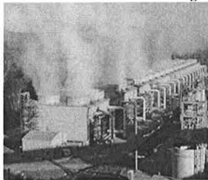
Figure 5. 40-cell Plant Yates cooling tower 25
