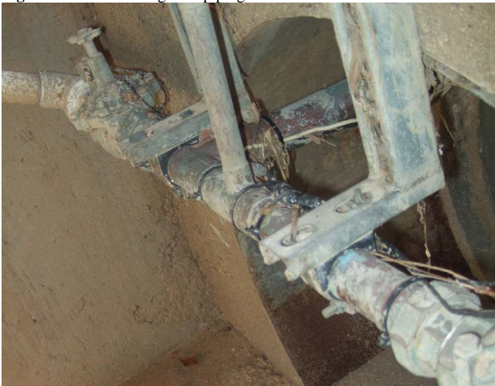
Figure 2-4. Private irrigation piping in storm drain
