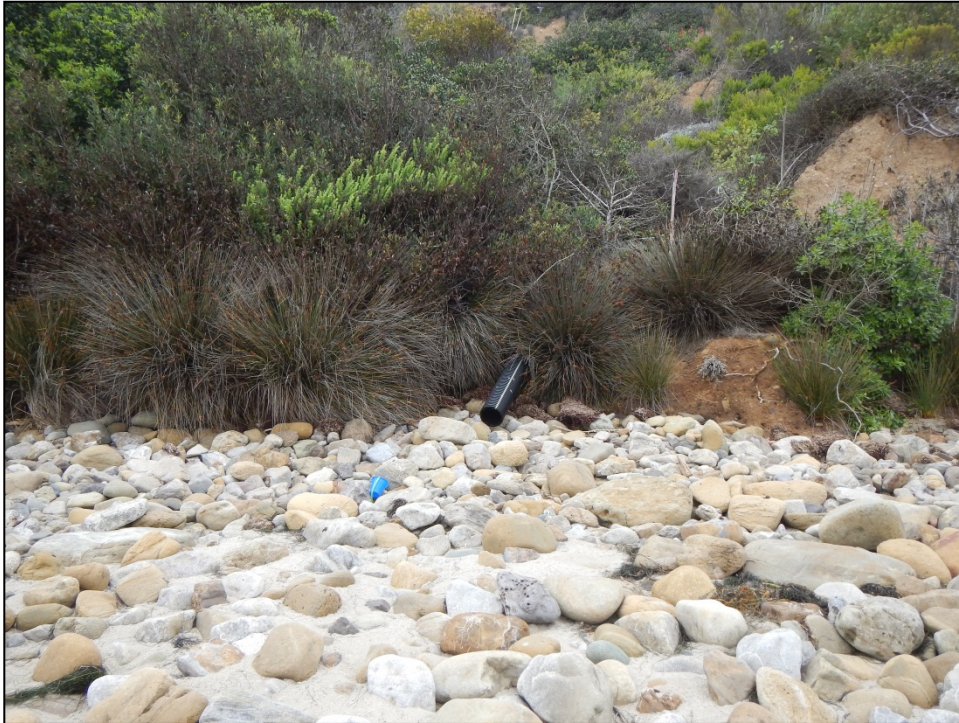
Figure 2-13. Typical Residential Small Drain Near La Piedra State Beach (ID #SAD375, 3-Inch Diameter)
