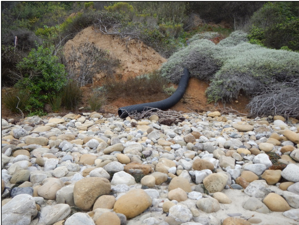
Figure 2-12. Typical Residential Small Drain Near La Piedra State Beach (ID #SAD379, 6-Inch Diameter)
