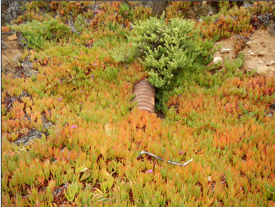
Figure 2-7. Small Drain End at Nicholas Canyon County Beach (ID #MUG091, 12-Inch Diameter)
