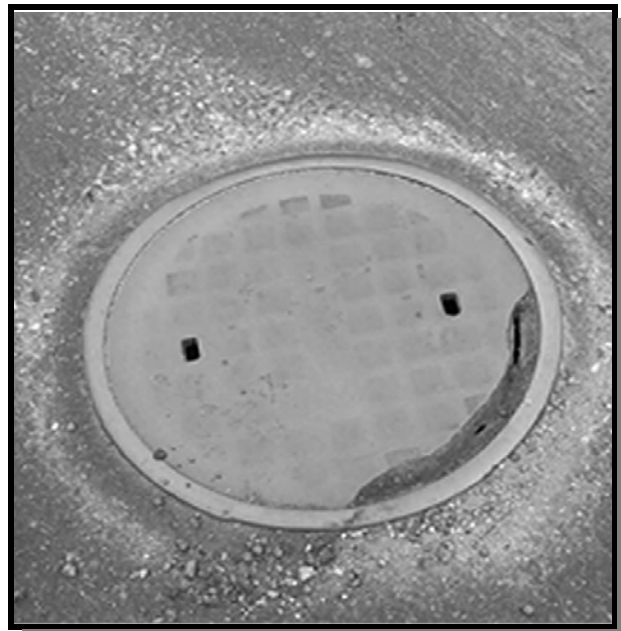
Damage to the sewer system infrastructure, such as this broken manhole cover allows stormwater into the sewer system (photo: Limno-Tech, Inc.)
