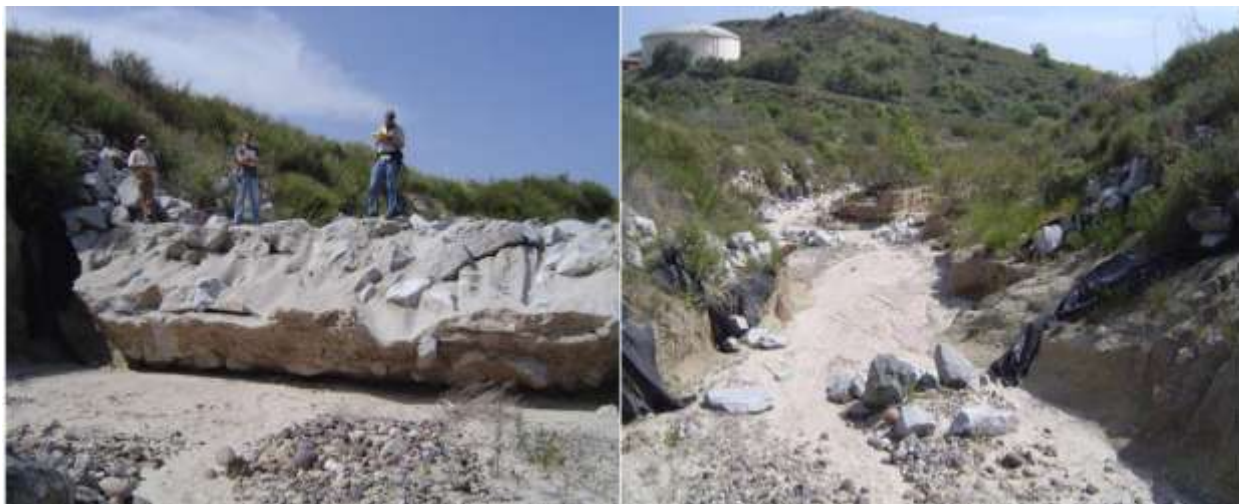
Figure 3-2. Undermining of grade control and erosion of banks downstream of structures intended to stabilize a particular stream reach. Left photo is looking upstream at drop structure; right photo is looking downstream from the drop structure.
