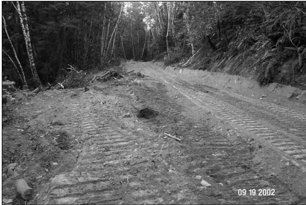
Figure X-D-26. Site # 5, 1312 Lower Road, before excavation. A potential road fill landslide was excavated at this site. Unstable outboard road fill was excavated and stockpiled locally along the cutbank behind the site, creating an outsloped road surface (see below).
