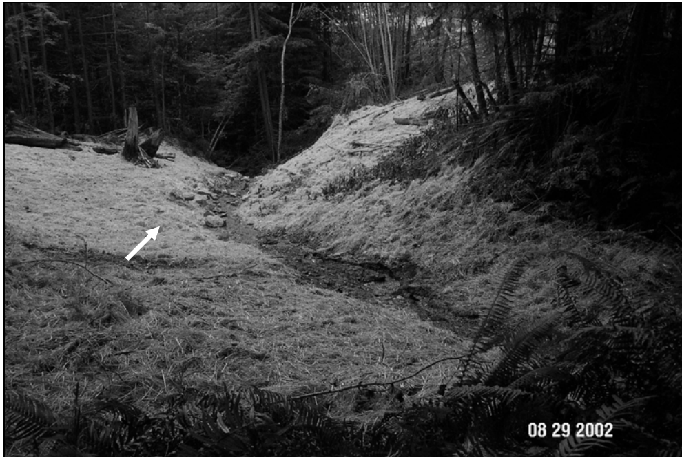
Figure X-D-10. Site #12, 1300 Road, after excavation. This picture was taken from the same viewpoint as Figure X-D-9. The stream crossing has been excavated, mulched and seeded. Upon excavation it was determined that the original watercourse meandered to the right prior to entering the Bot. Armor was placed along the left bank to prevent stream bank erosion (see arrow).
