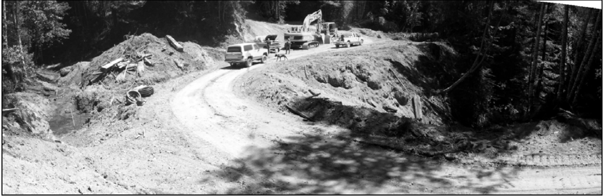
Figure X-D-18. Site #3, 1311 Road, before excavation. This is a 3 shot panoramic compilation photo taken from the cutbank on the right approach to this Humboldt stream crossing. The site has been brushed out and a temporary flex pipe has been installed along the right hinge line to divert active flow around the work area.
