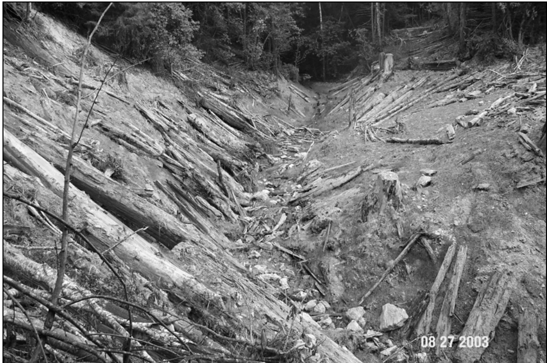
Figure X-D-23. Site #3, 1311 Road, after excavation. This picture was taken from near the right bank looking upstream.
