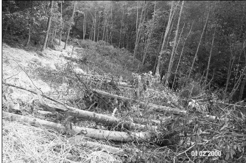
Figure X-D-25. Site # 2, 1312 Lower Road, after excavation. This picture was taken from the same viewpoint as above. The unstable road fill has been completely excavated, mulched and seeded, leaving an outsloped road surface. Note trees and brush removed during excavation have been used a ground surface mulch. Panther Creek (not visible in photo) is located to the right.
