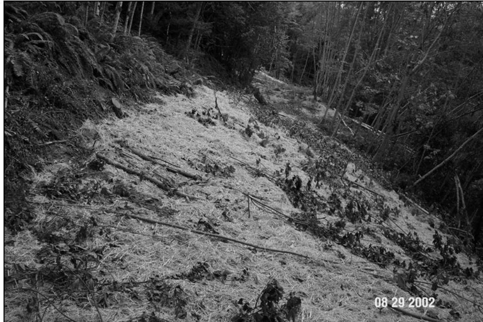
Figure X-D-12. Site #10, 1305 Road, after excavation. This picture was taken from the same viewpoint as Figure X-D-11. The unstable road fill has been completely excavated, mulched and seeded, leaving an outsloped road surface. Because this road exhibited nearly continuous road fill instabilities, a similar nature of treatments were applied to the remaining road, along with stream crossing excavations.
