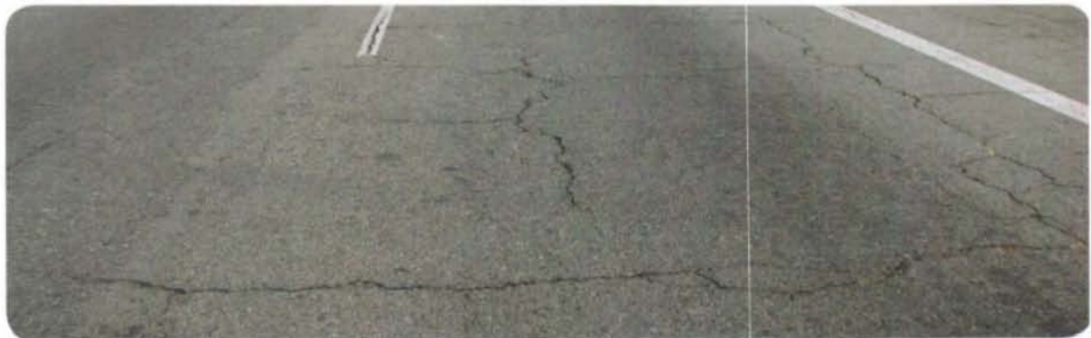
Main - 28th to 29th, Pavement Condition Index 43, Grade D
