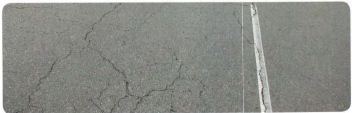
Figueroa & 48th, Pavement Condition Index 57, Grade C-
