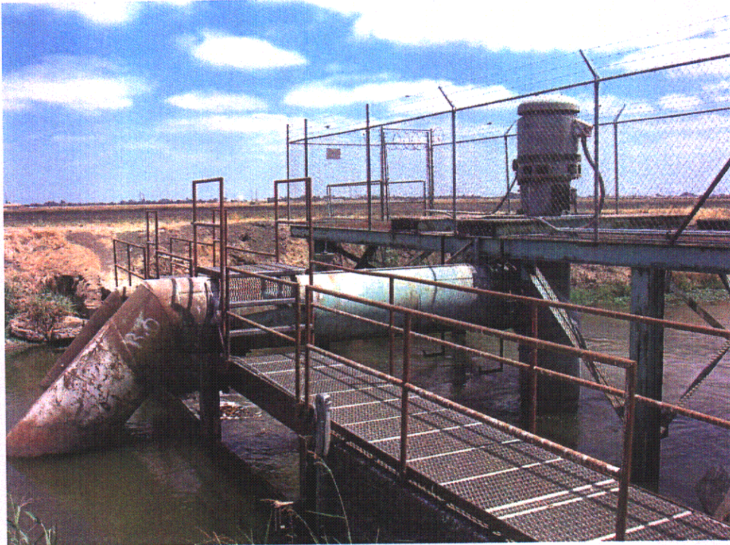
POINT E to POINT F - Elkhorn Lift Station (East Drainage Canal)
