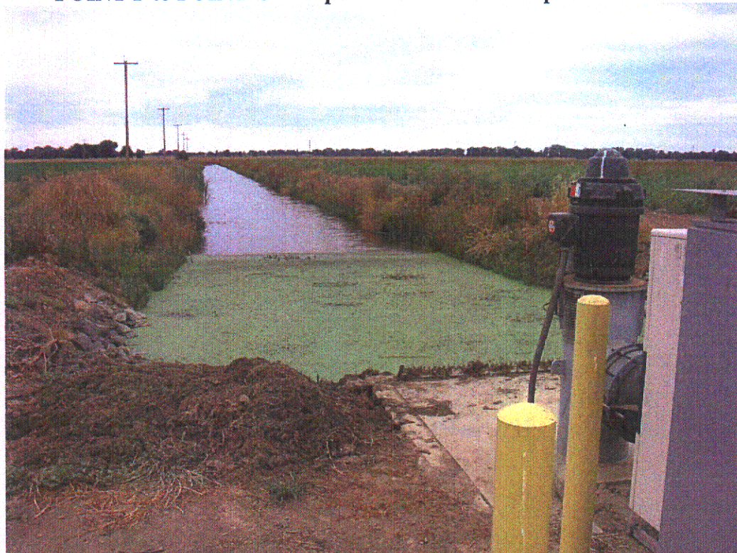
POINT F to POINT G - Airport/Bayou Lift Station (Off West Drainage Canal) – View South
