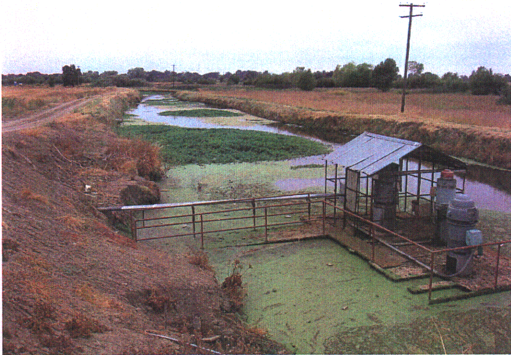
POINT E to POINT 2 - Pullman Lift Station – View Southwest
