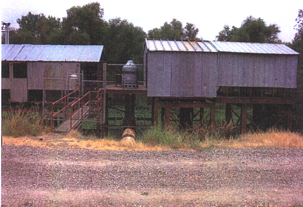
POINT B - Northern Pumping Plant (Natomas Cross Canal)
