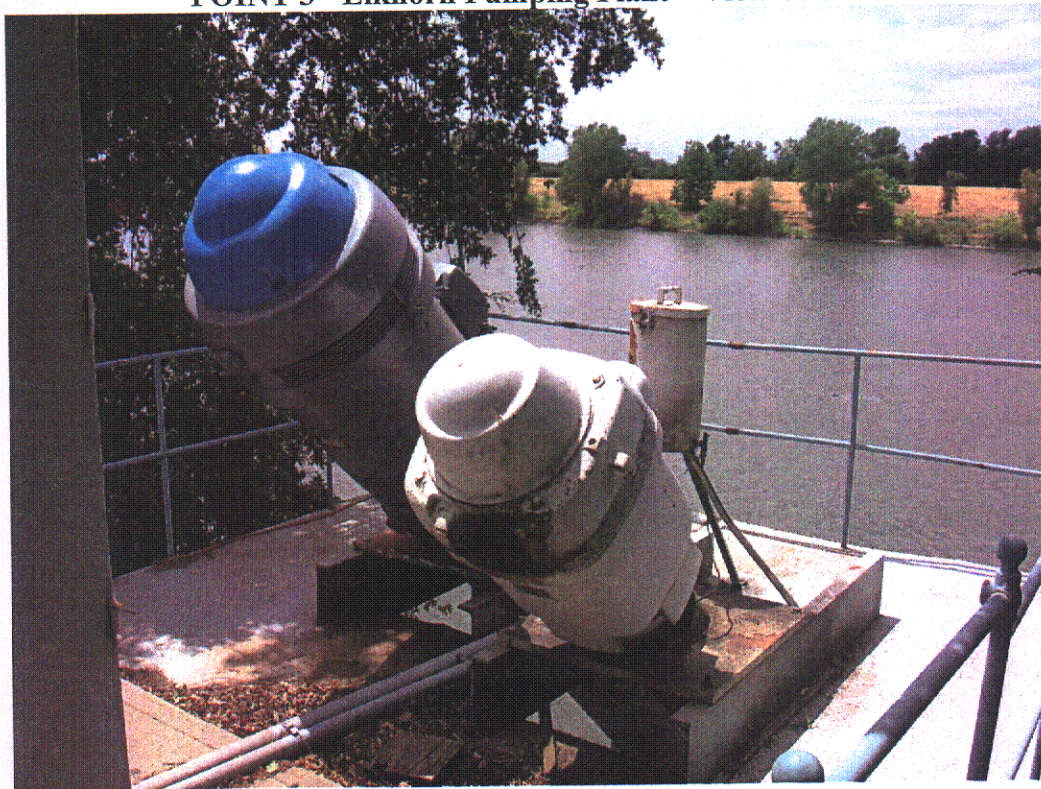
POINT 6 - Riverside Pumping Plant (Sacramento River)
