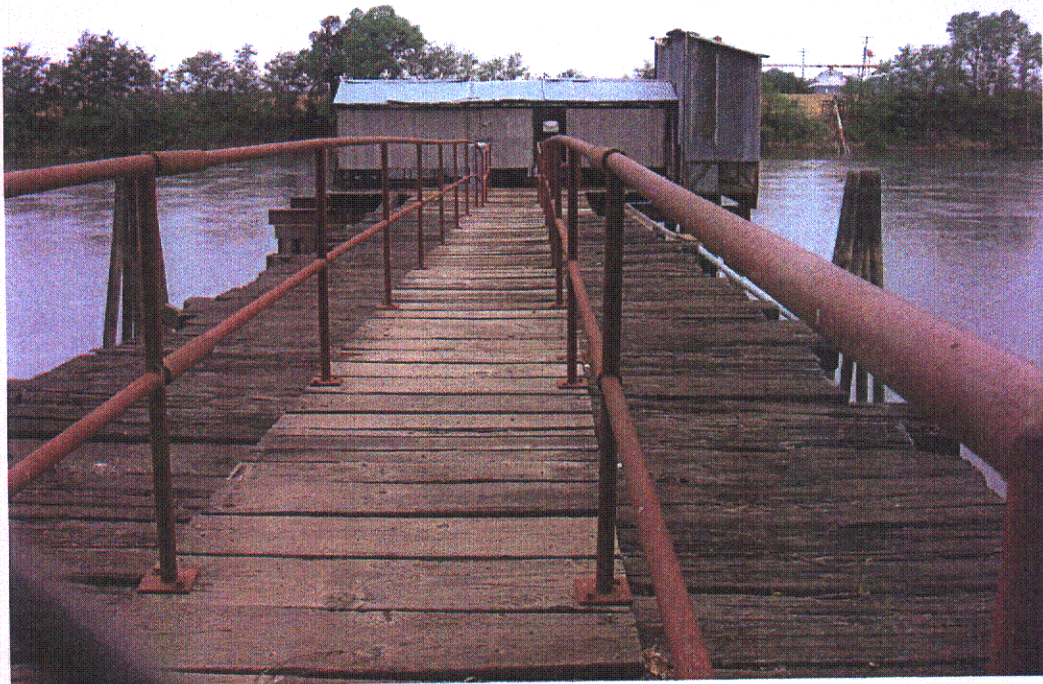
POINT 2 - Pritchard Lake Pumping Plant (Sacramento River)
