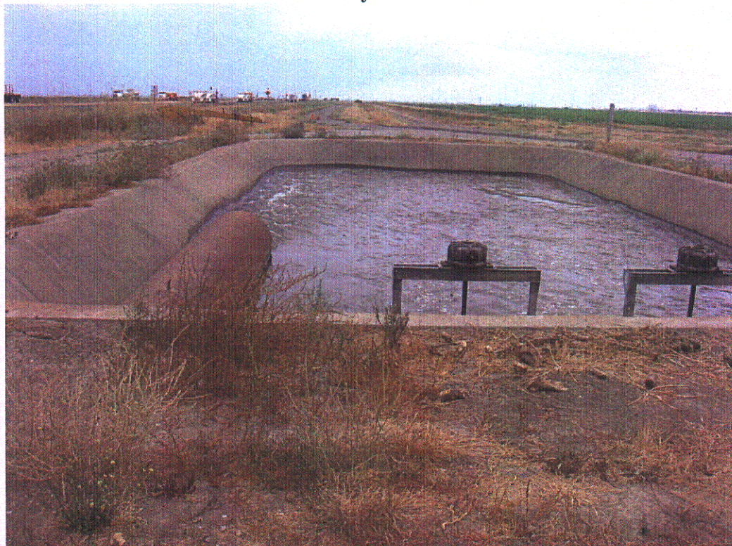
POINT E to POINT F - County Line Lift Station – View North
