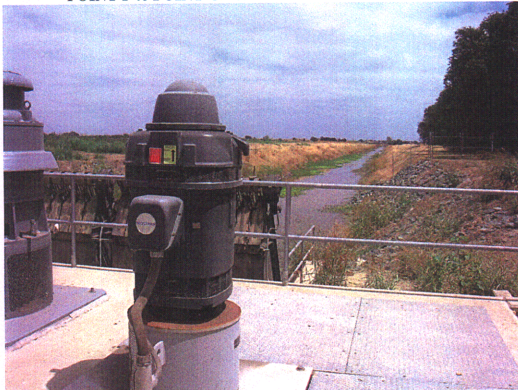
POINT F to POINT G - Plant 3 Pump (Off West Pumping Plant) – View East
