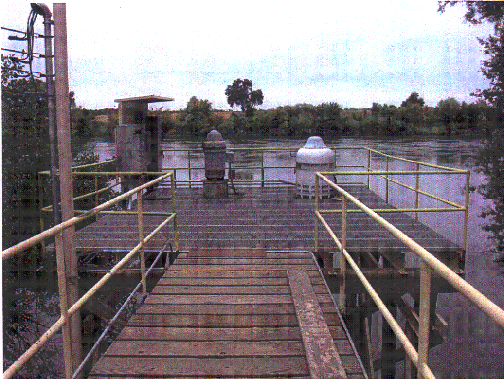
POINT 3 - Elkhorn Pumping Plant (Sacramento River)
