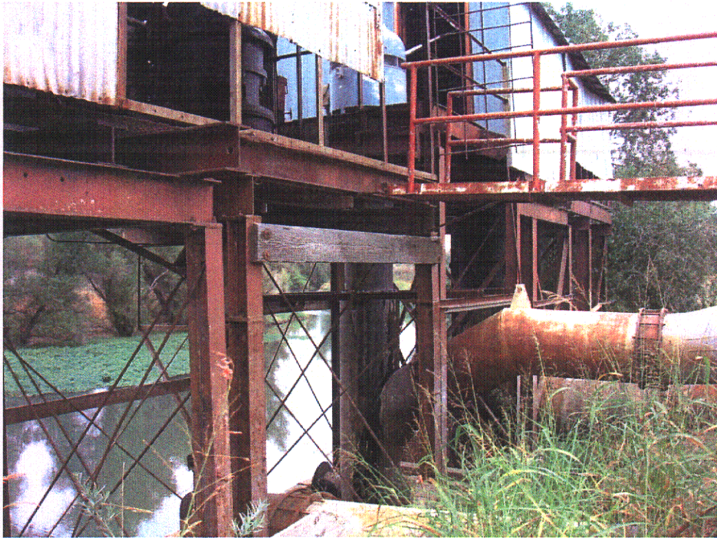
POINT B - Northern Pumping Plant – View Northeast
