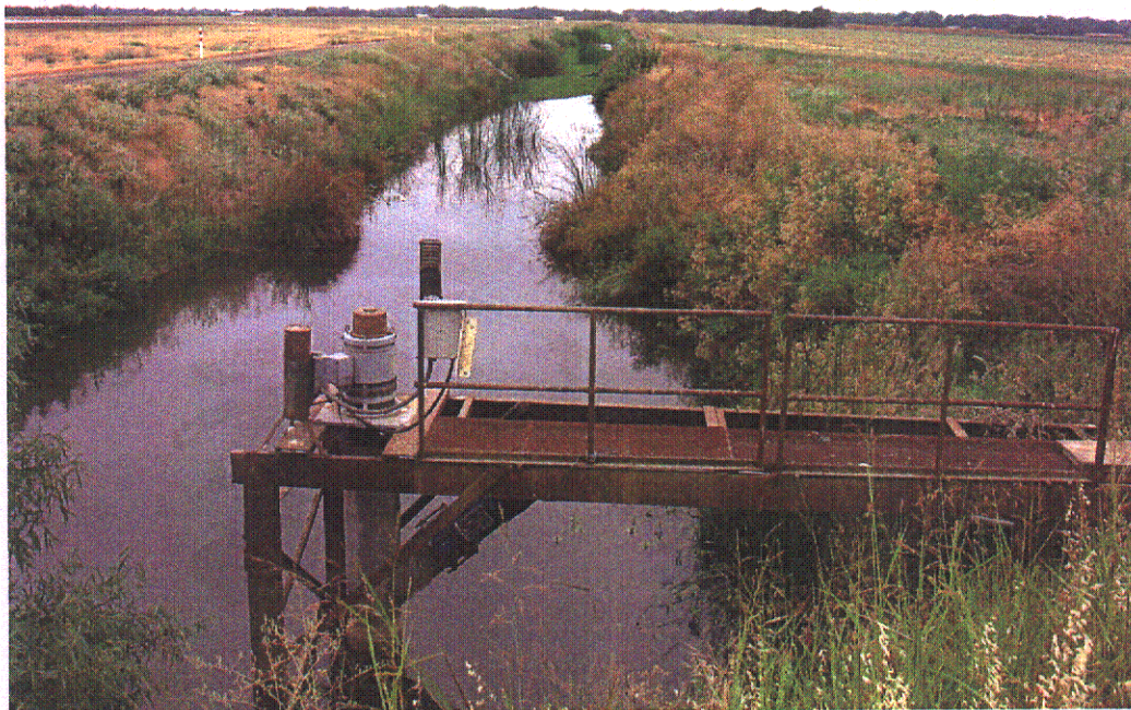
POINT F to POINT G - Airport North Drain Pump (Off West Drainage Canal) – View South
