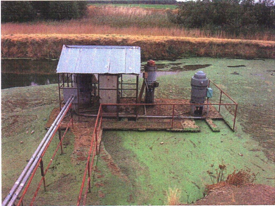
POINT E to POINT 2 - Pullman Lift Station (Confluence of North and Central Main Canals)
