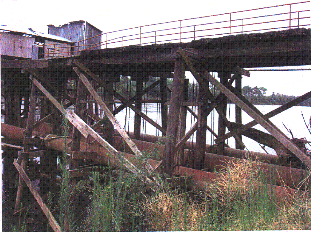
POINT 2 - Pritchard Lake Pumping Plant – View North
