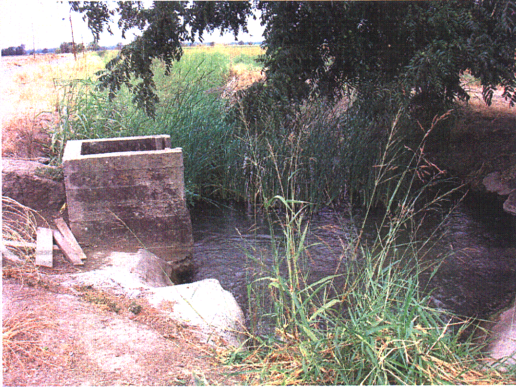
POINT F to POINT G - Rosa Drain Pump— View West
