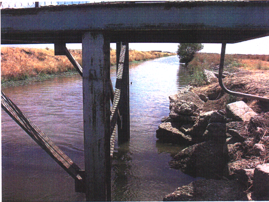
POINT E to POINT F - Elkhorn Lift Station – View South
