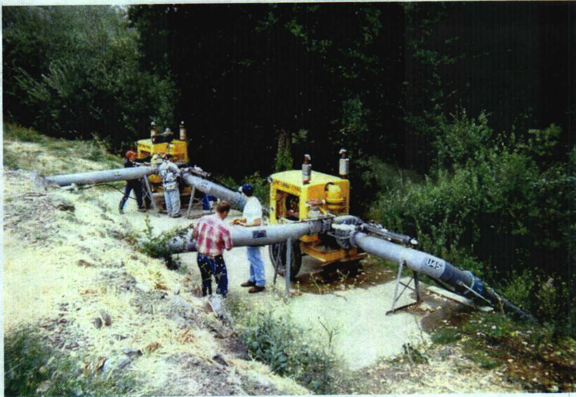
Two Cornell pumps powered by International engines that are fueled with natural gas at the point of diversion.
