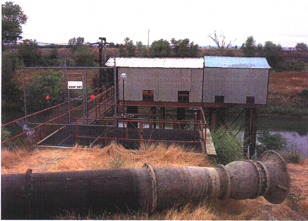
POINT A - Bennett Pumping Plant (Natomas Cross Canal)
