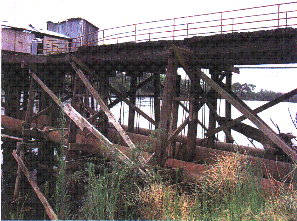
POINT 2 - Pritchard Lake Pumping Plant – View North
