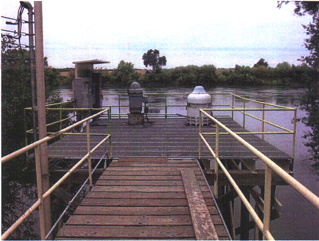
POINT 3 - Elkhorn Pumping Plant (Sacramento River)
