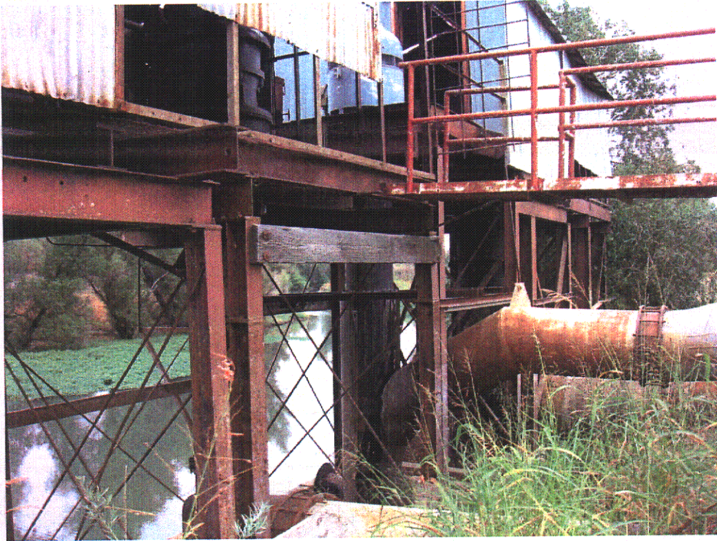
POINT B - Northern Pumping Plant – View Northeast
