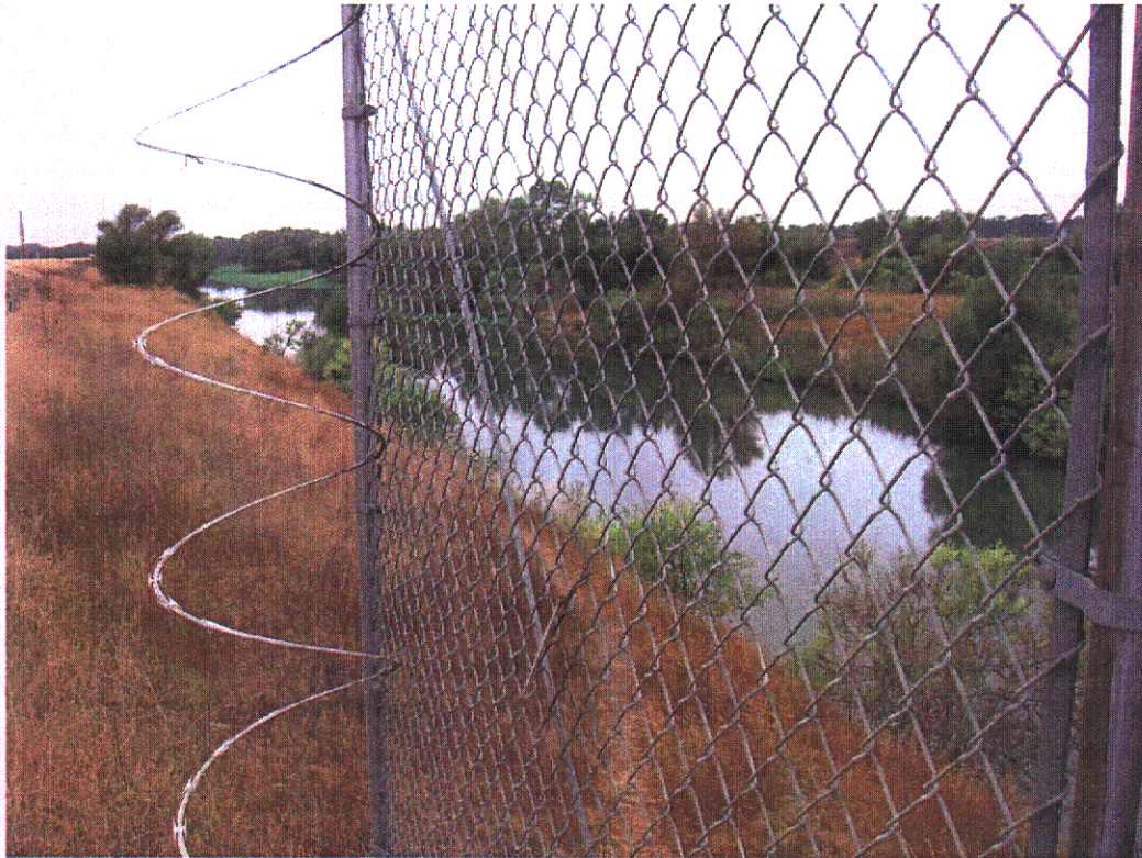
POINT A - Bennett Pumping Plant - Southwest
