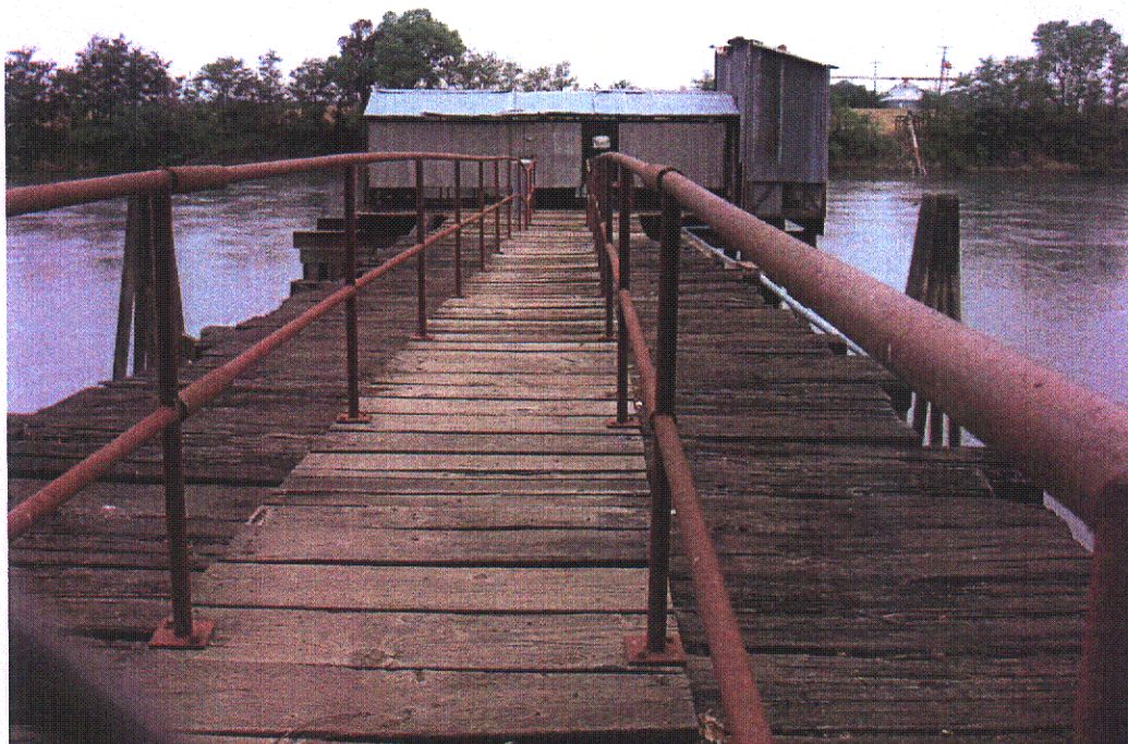
POINT 2 - Pritchard Lake Pumping Plant (Sacramento River)
