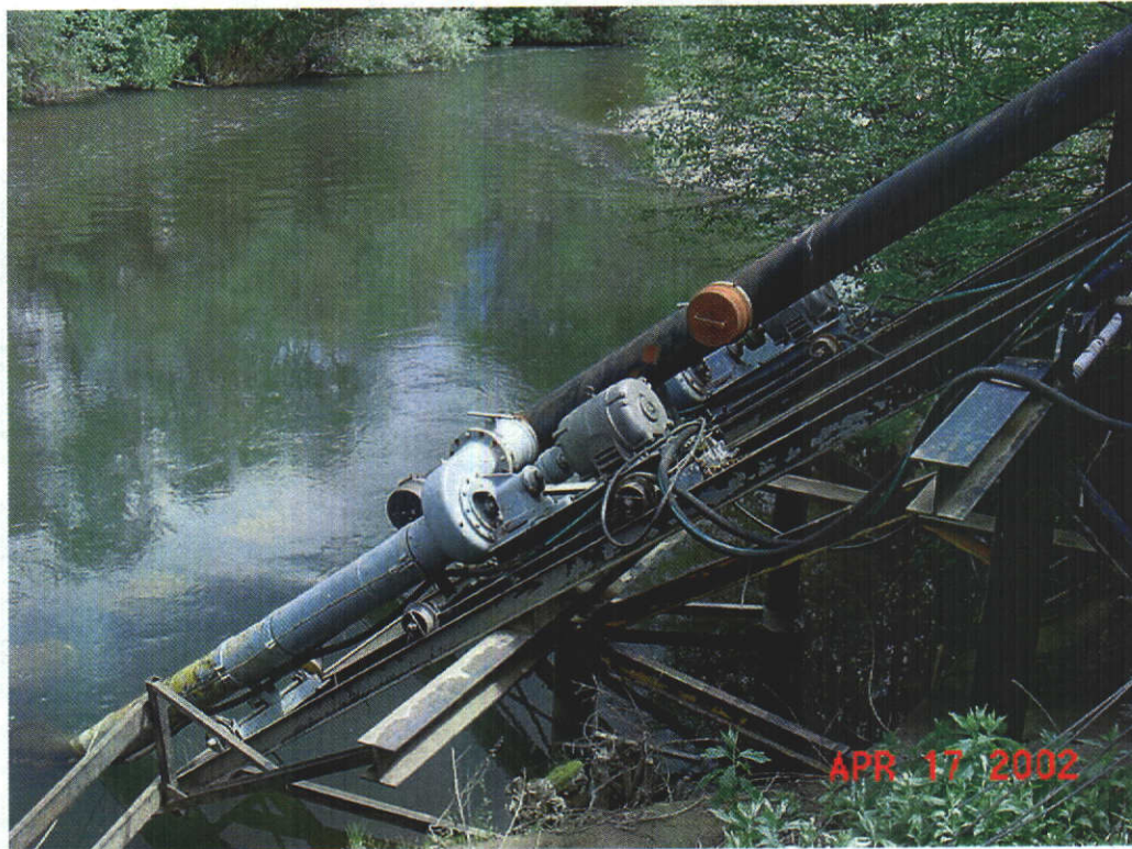
Electric pumps used to stabilize pumping head in the sump
