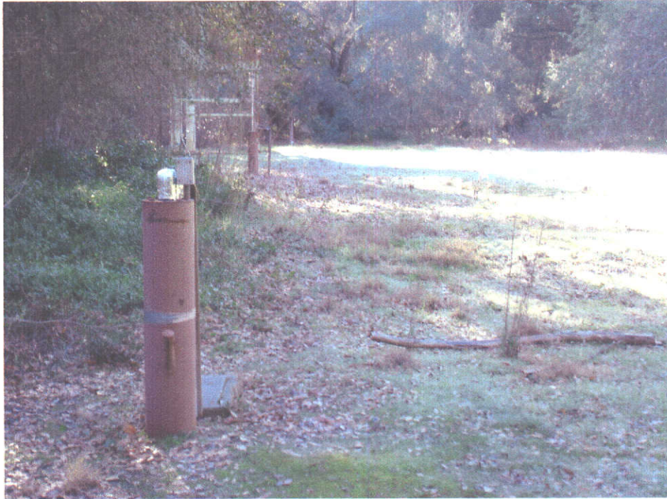
Photo showing the Riverside Well Field—Wells #1-#4 are seen in photo looking south. (Well #2 is in foreground, Well #4 is in background) Note dense riparian vegetation to left (east) of wells.
