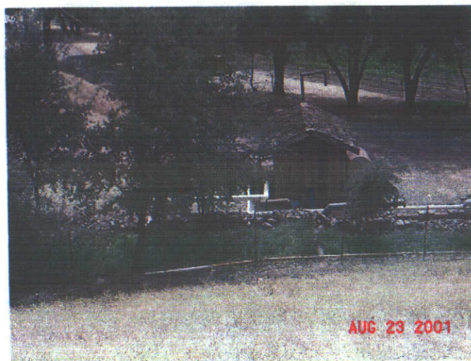
Pump house at the base of the dam at the "Back" Reservoir.
