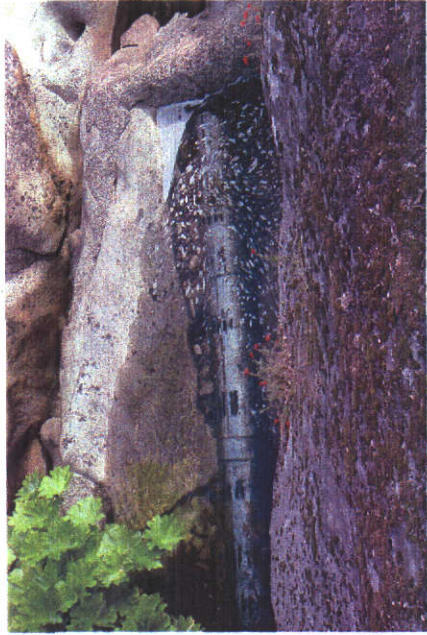
Concrete berm constructed over downstream side of intake screen to help pool water.
