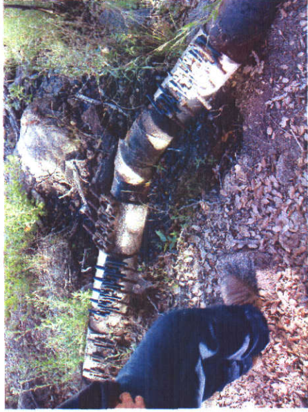
Multiple repairs over a short distance.
