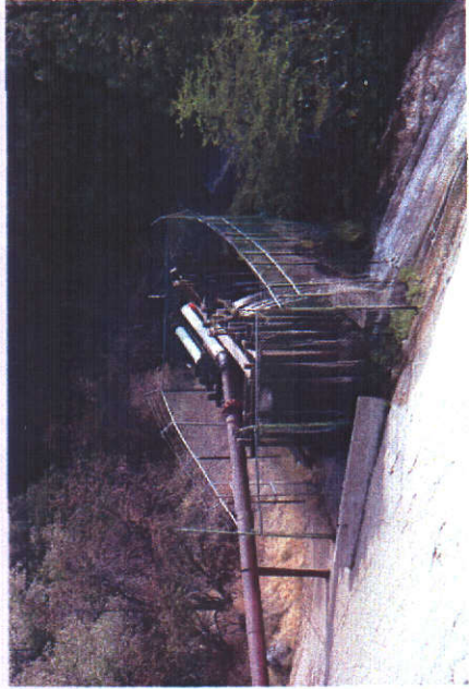
2-stage sedimentation boxes
