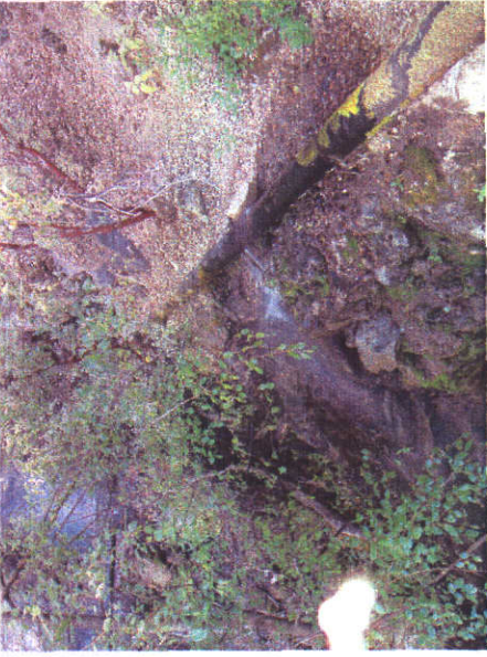
More damaged pipe downstream of intake.
