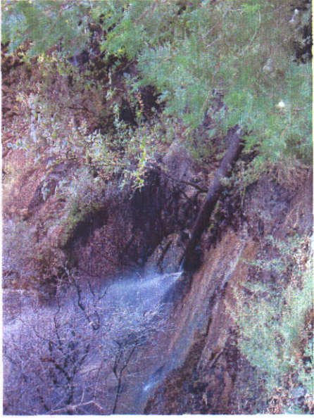
Damaged pipe just downstream of intake.
