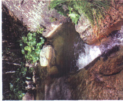
View of intake pool taken from upstream. The date of this photo is 8/19/08.
