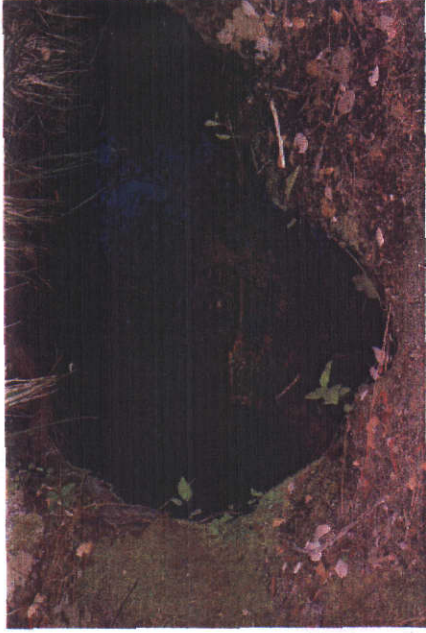
Pool created by leak in underground portion of pipe.
