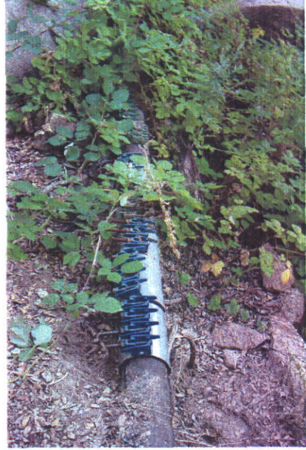
Multiple repairs over a short distance.
