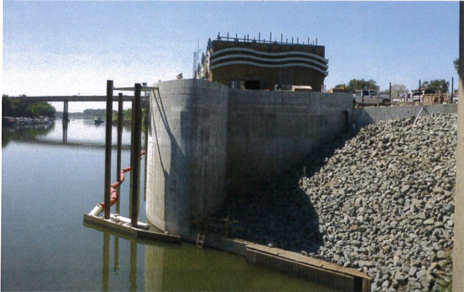
View of the new joint intake facility facing south (downstream) from the existing RD 2035 intake (June 28, 2016)
