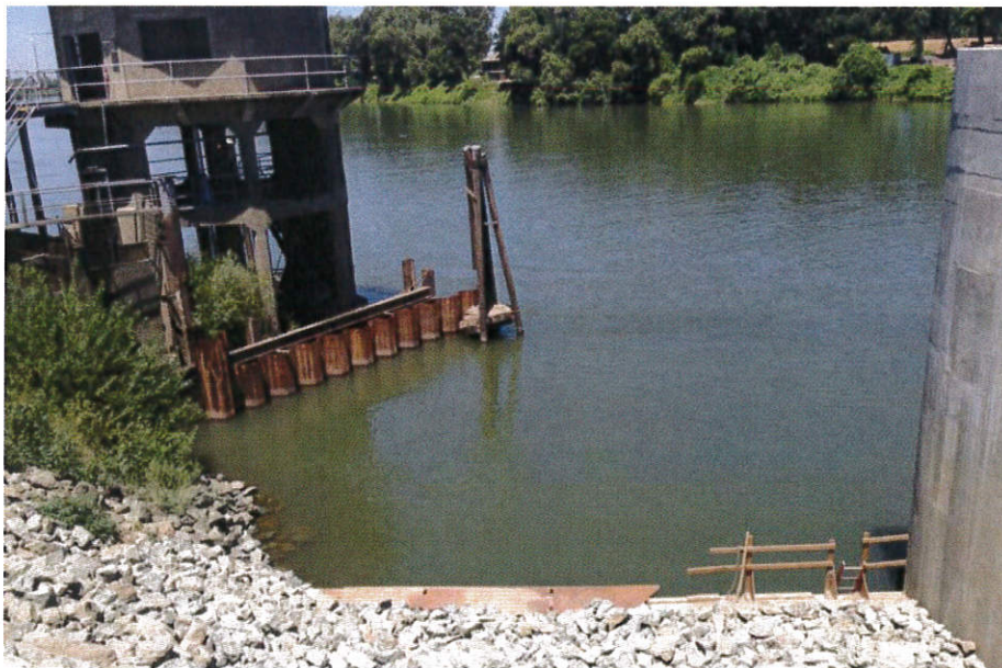
View of the existing RD 2035 intake facing north (upstream) from the joint intake facility (July 12, 2016)
