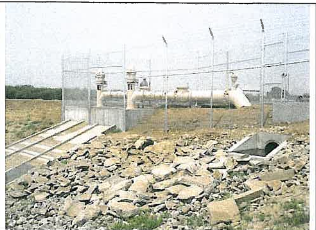
Reservoir pump station. Tailwater will enter the reservoir through the pipeline outlet (foreground) and recirculated into the irrigation system through the pump station.
