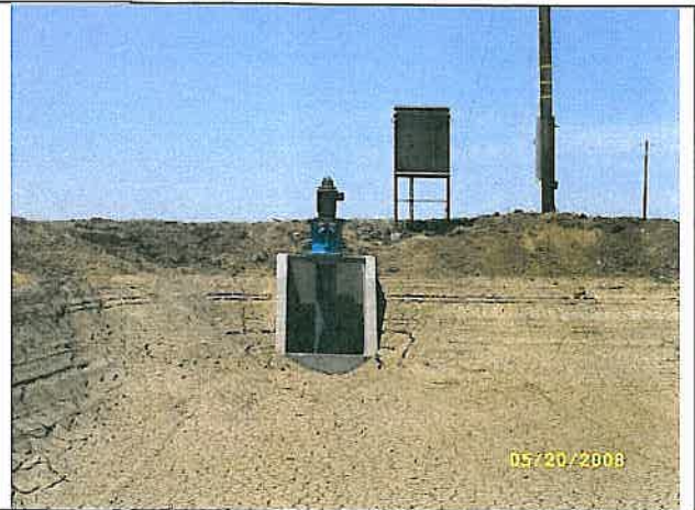
Westley Tailwater Pond – Pump station in the primary basin.
