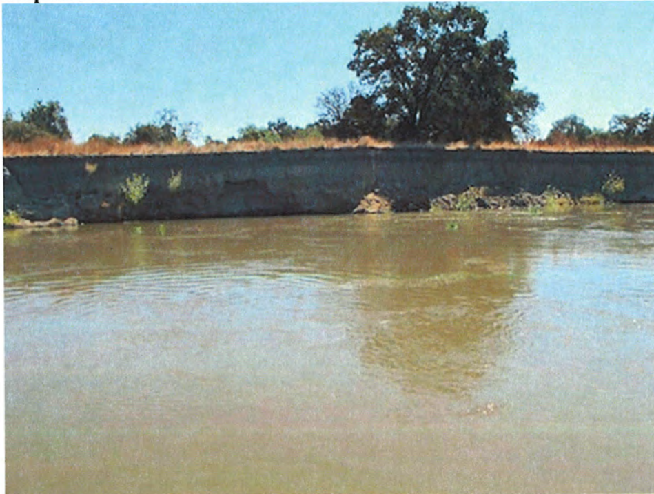
Figure 12. In some areas of the lower San Joaquin River, the steep levees have begun to erode.
