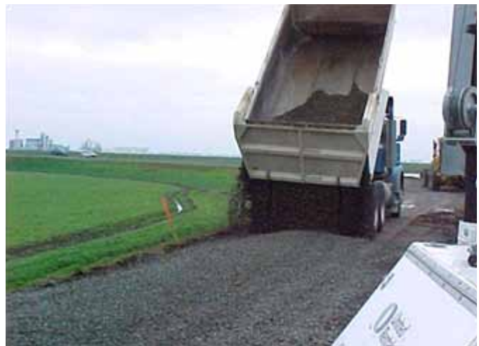
To quickly respond to flood emergencies, the State proposes to provide all-weather access roads on levee crowns
