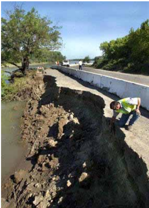
Erosion along the Sacramento River
