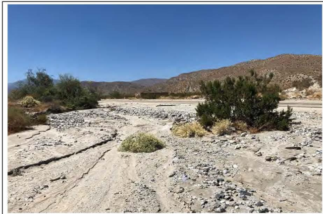
Photograph 15: View to the north (upstream) of Drainage P that flows across North Indian Canyon Drive at Big Morongo Siphon [Work Area 24].
