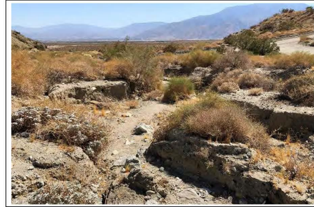
Photograph 10: View to the south (downstream) of Drainage K located at Big Morongo Siphon [Work Area 24].
