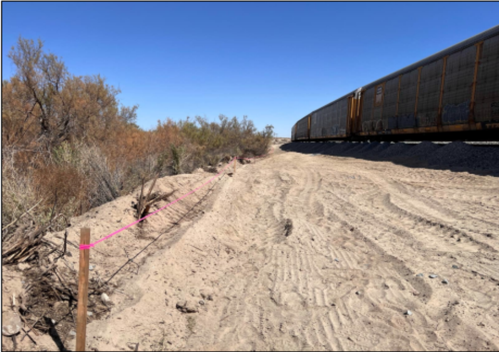
Photo 1. Northeast side of track repair fill area adjacent to Wetland North. Note avoidance flagging.
