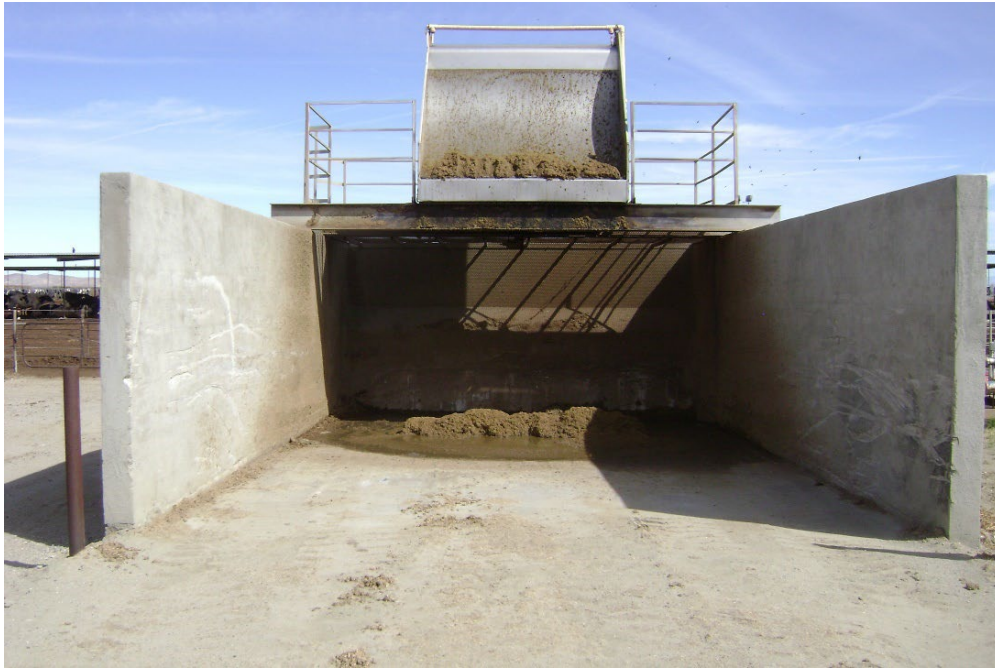
Photograph 5—Separator device to remove manure solids from dairy parlor wash water.
