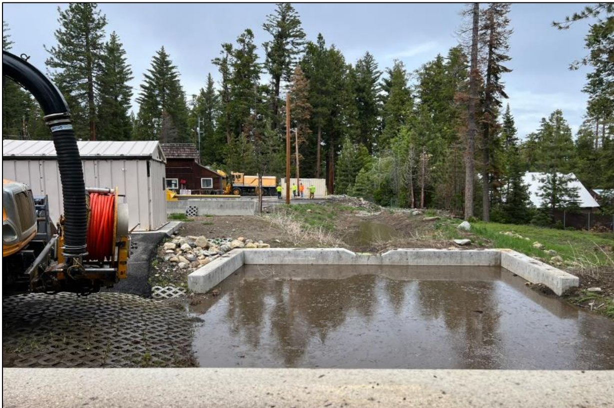
Photo 2.1: As part of maintaining stormwater infrastructure, Vactor trucks are used to clean sediment out of sand traps, culverts, and rock-lined swales. Here, a Vactor truck is shown transferring material to a decanting facility. El Dorado County Yard inspection, June 12, 2023.
