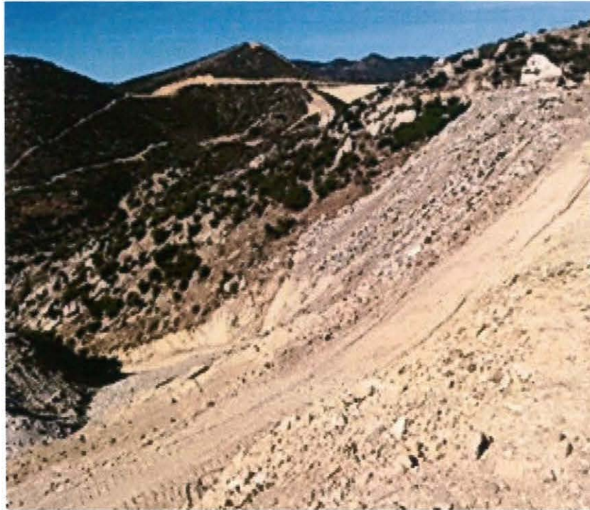
Figure 8. View facing west of the stockpiling areas where fill (construction debris) has been discharged into the tributary, filling the canyon from the top. Also, graded road area heading further south into the canyon.
