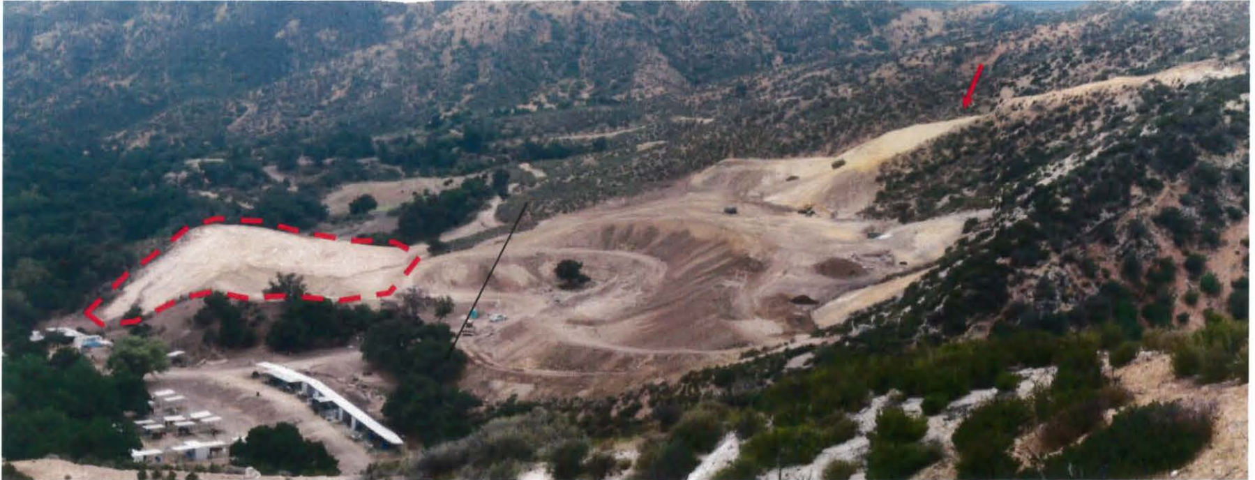
Figure 4: Panaoramic view looking south from the Browns Canyon Road at grading/fill operations in the parcel 2821-009-030, 2821-009-031 area. The dashed line is the approximate boundaries of a large area (proposed horse arena) not included in the initial grading plans and is encroaching towards Ybarra Creek. Grading for new access to the area (arrow) was also not included in the initial grading plans.
