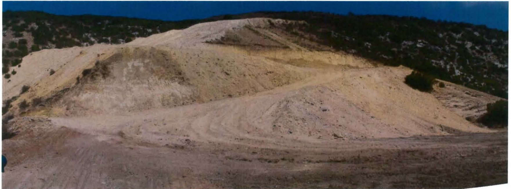
Figure 7: View of a road being graded to provide new access to 2821-009-030 and 2821-009-031 parcels that was not included in the initial grading plans.
