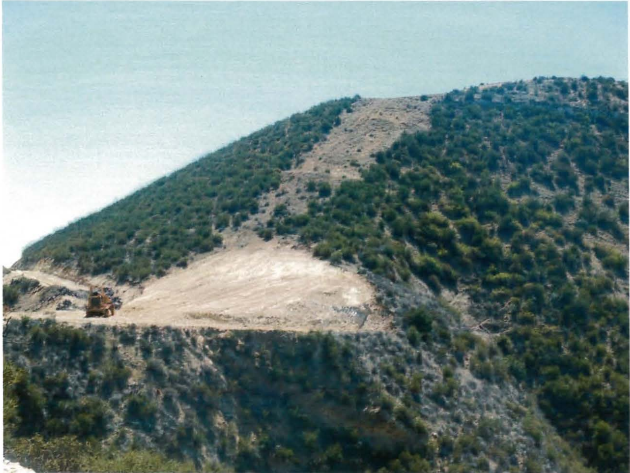
Photo 16. This photo shows the top area of ongoing grading activities shown in photo 10, above.
