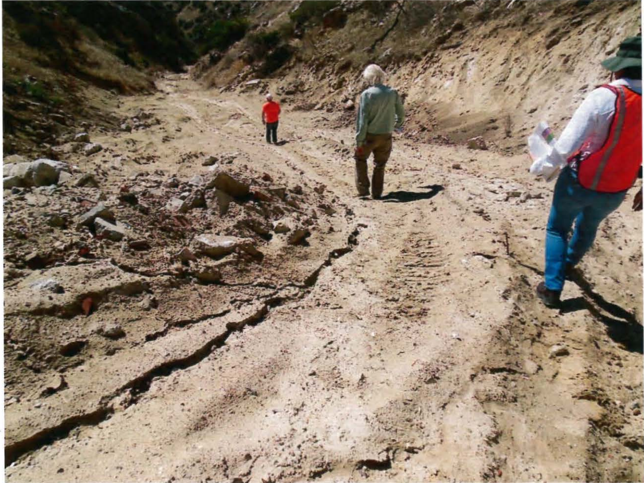
Photo 6. This photo shows the ravine immediately down gradient from the waste stockpile that leads to Ybarra Creek. Note the steep gradient, loose sediment, and rills.
