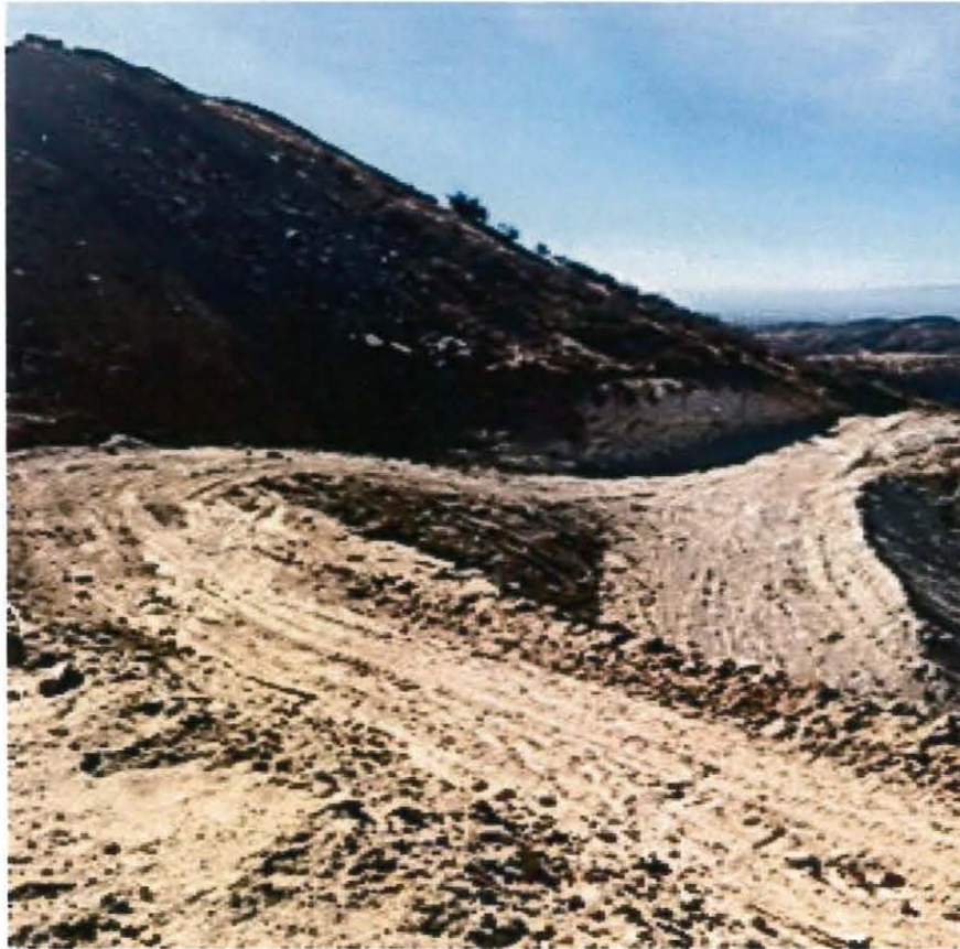
Figure 5. View from the unnamed tributary toward the east, depicting areas which have been graded into access roads to fill portions of the tributary below.
