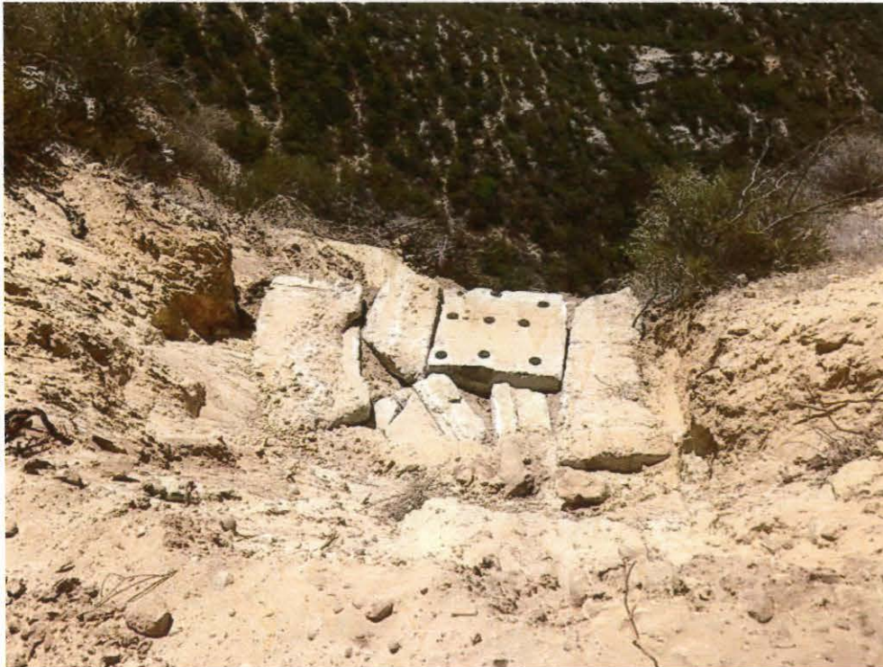
Figure 10. Area where filling of the slope has begun. The ravine below is a tributary to Devil's Canyon. (LB Nye)
