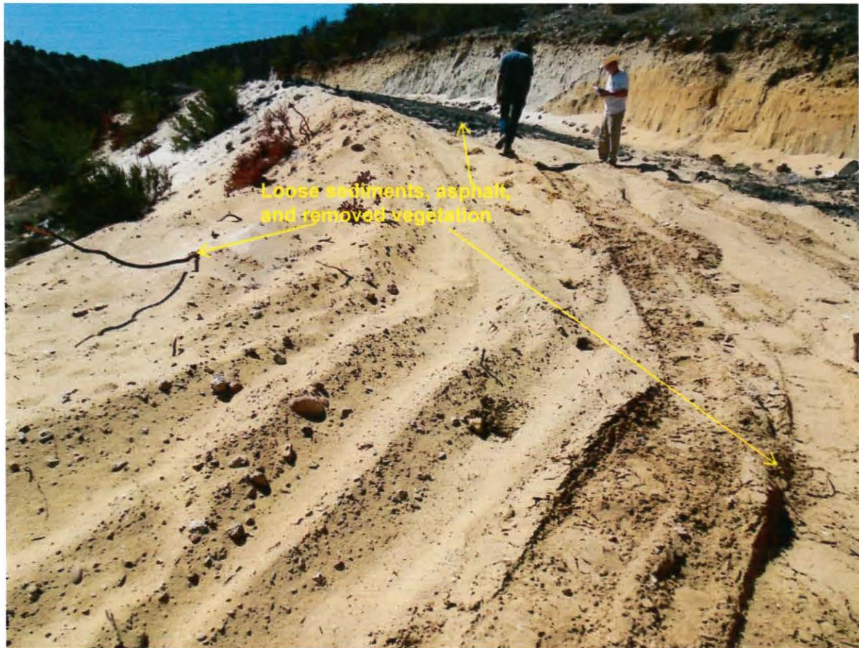
Photo 13. This photo shows graded area 3 with loose sediments, and removed vegetation. Weathered asphalt debris is being used locally to armor/stabilize the roadway.
