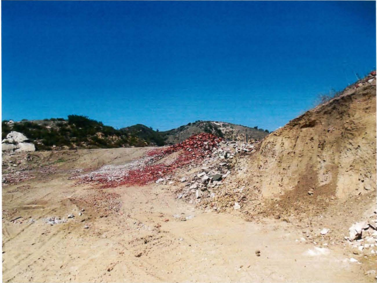
Photo 4. Graded area 2 with stockpiled of pieces concrete, brick, tile, and other debris.
