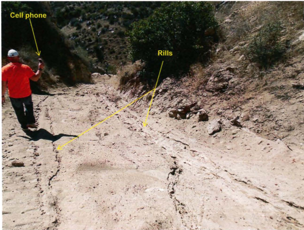
Photo 7. This photo is of Mr. Todd Fishback recording the inspection using his cell phone. In addition, the photo shows rills along the slope flooring the recently graded ravine from the top of the graded area 2 down to a sediment basin (shown in photo 8) above Ybarra Creek.
