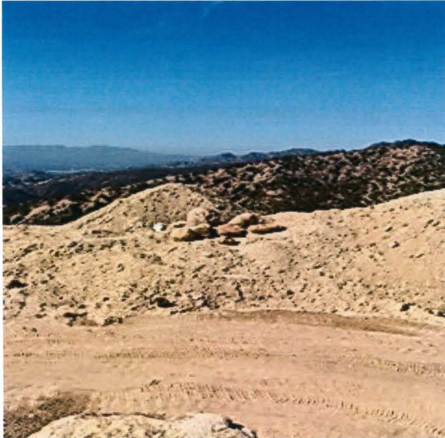
Figure 13. Graded road and stockpile on top of the eastern slope above the unnamed tributary to Brown's Canyon.
