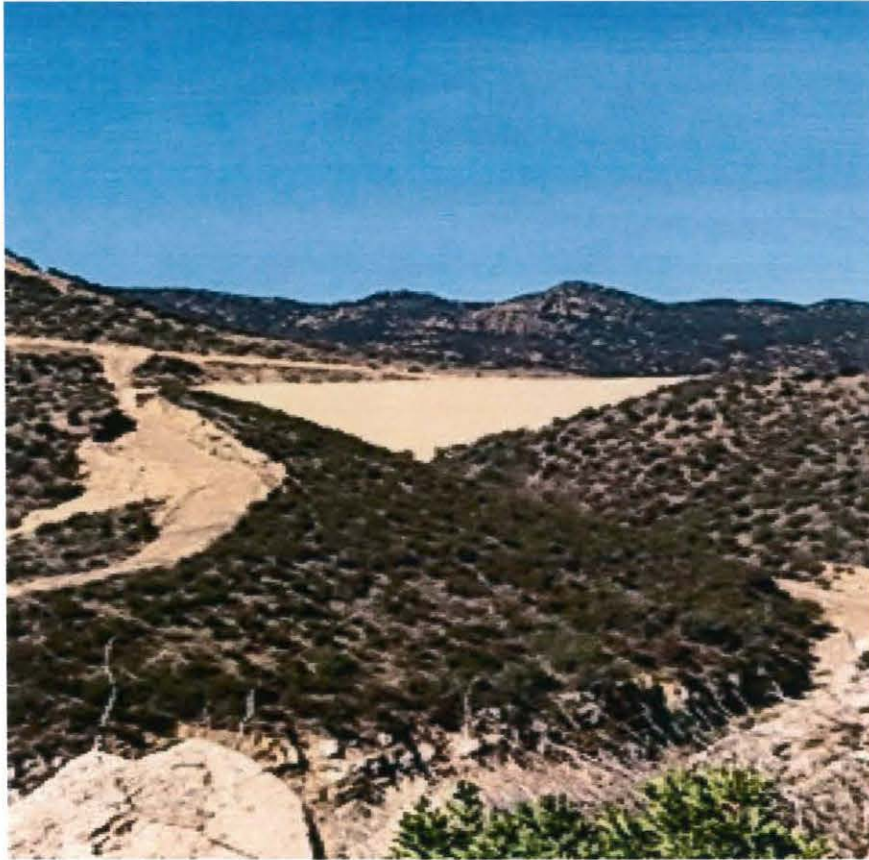
Figure 11. View facing west of the graded slope and the fill material that was placed to construct the berm for a road.
