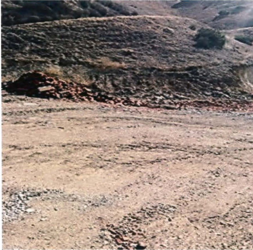
Figure 3. View of the top of the graded area of the canyon. Stockpiled materials on the eastern side of the graded slope.
