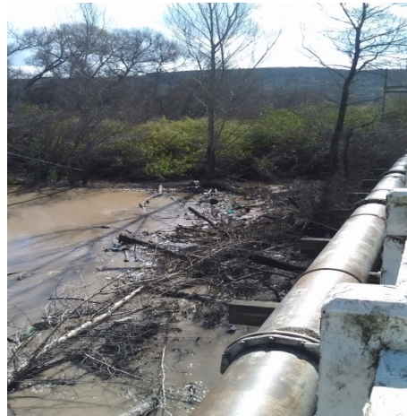
Dead trees against Hollister Street Bridge footings.
