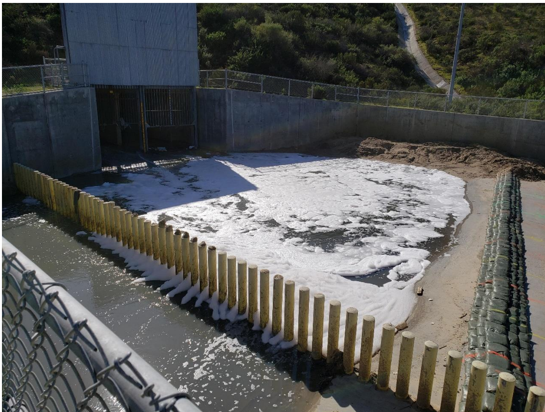
Figure 6: Smugglers Gulch Diversion Structure on January 22, 2020, Photo by Customs and Border Protection
