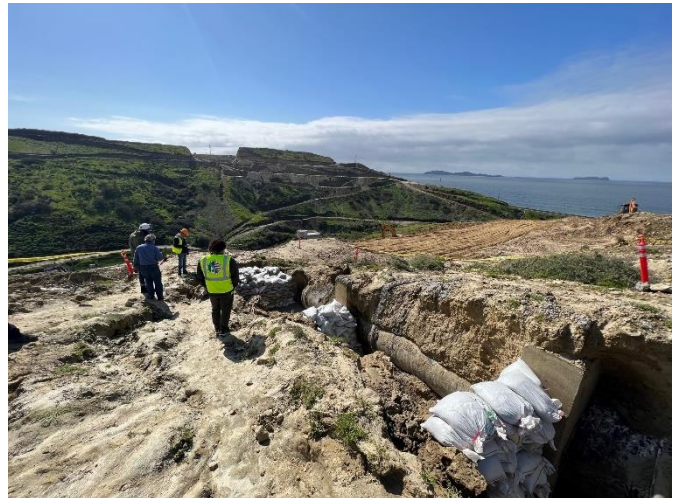
Photo 2: Inverted Siphon No. 4 Land Erosion (La Joya)
