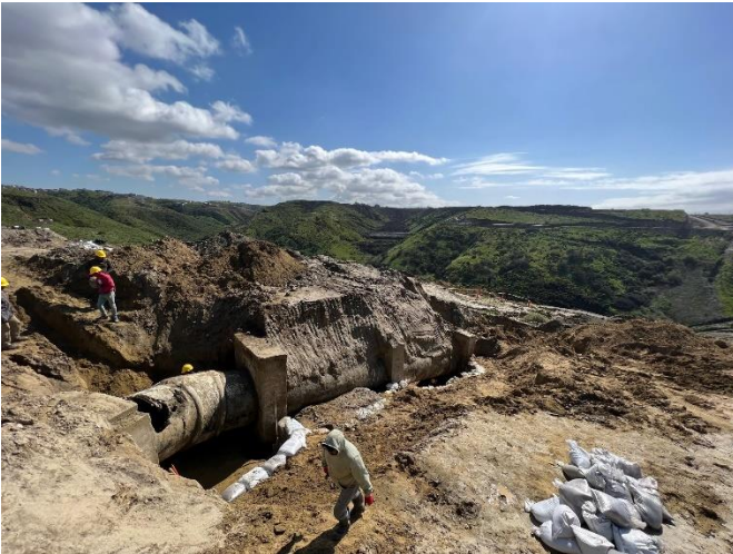
Photo 1: Inverted Siphon No. 4 Land Erosion (La Joya)
