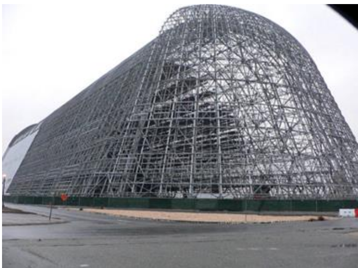
Figure 1b: Hangar 1, to be resided by Planetary Ventures as a requirement of its lease with NASA.
