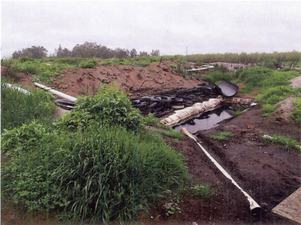
3/3/2016 – Storm water management system.
