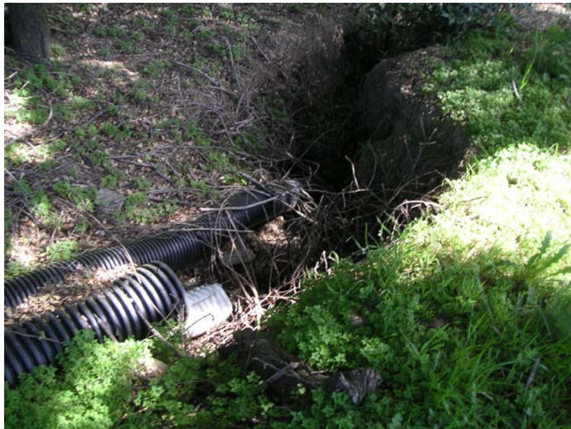
Figure 3. Gully Formed by Discharge of Concentrated Runoff from Hillside Vineyard
