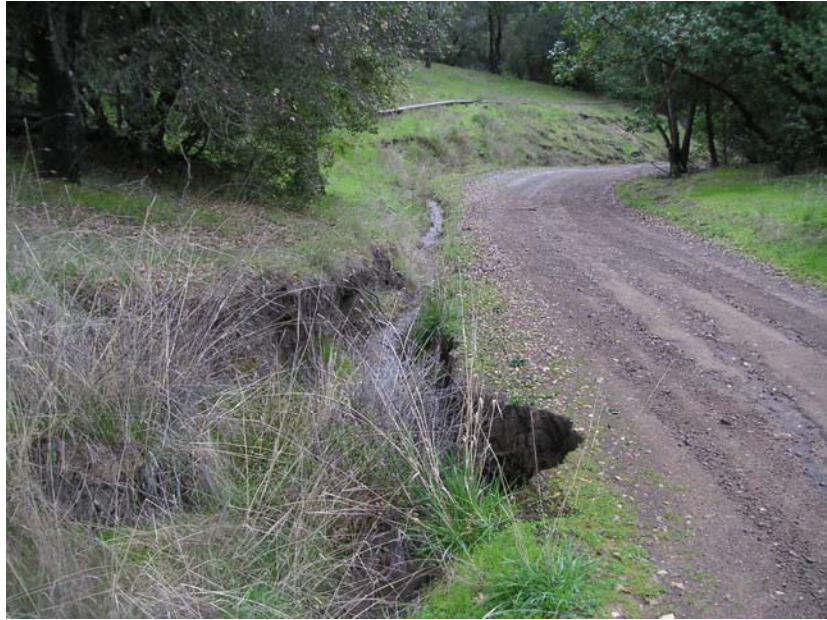
Figure 4. Rills and Gullies on a Compacted Dirt Road Gully forms where runoff depth and slope are sufficient to erode soft colluvium at this site, which is underlain by the m \acute{e} lange bedrock unit.
