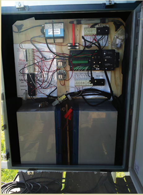
Figure 5. Electronics inside a flow-station gage house.
