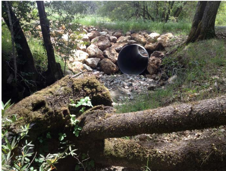
PWA Site #6 inlet
