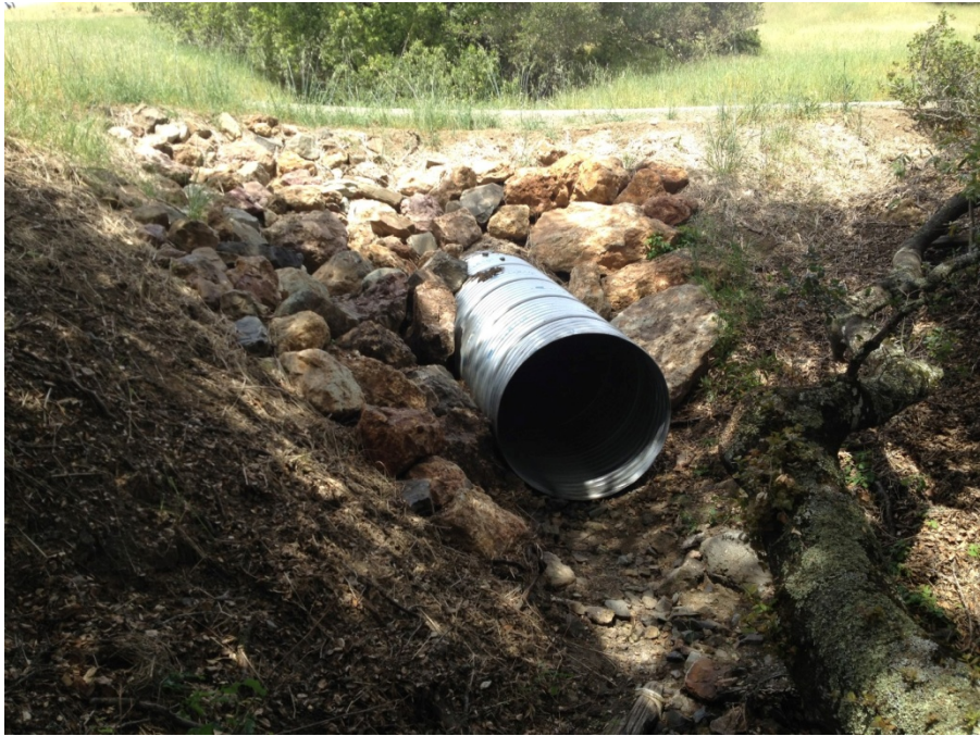
PWA Site #5 inlet
