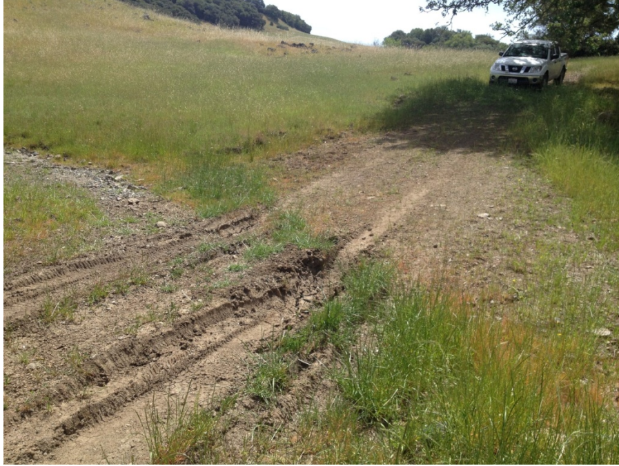
PWA Site # 33 – Tire ruts in road
