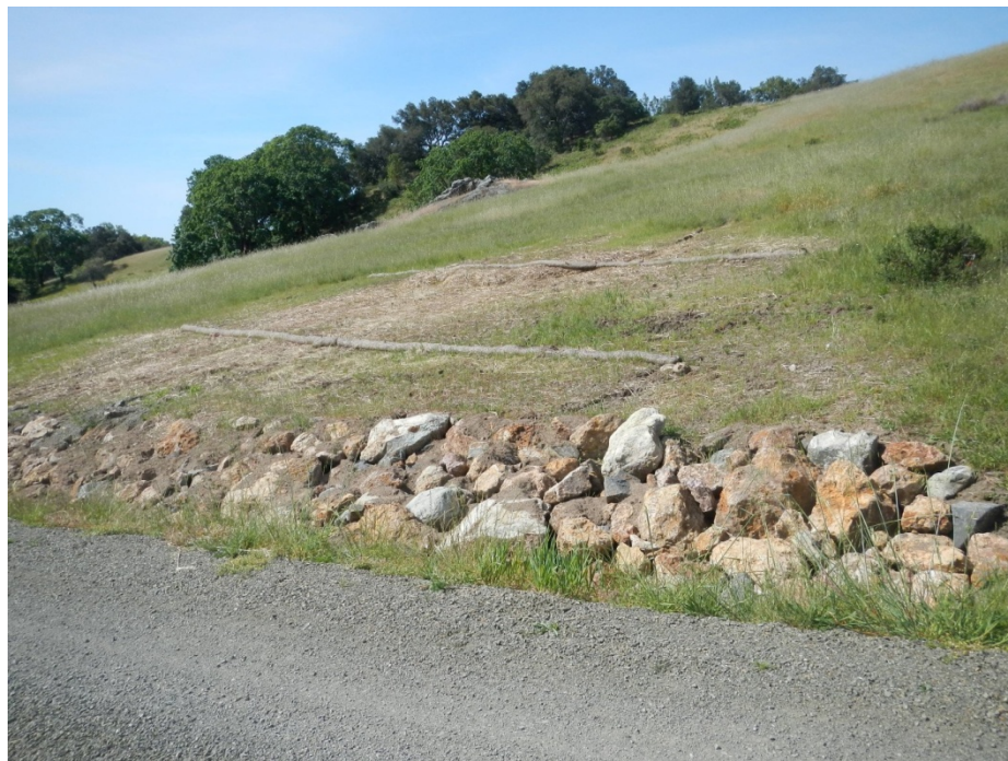
PWA Site 7.2 landslide
