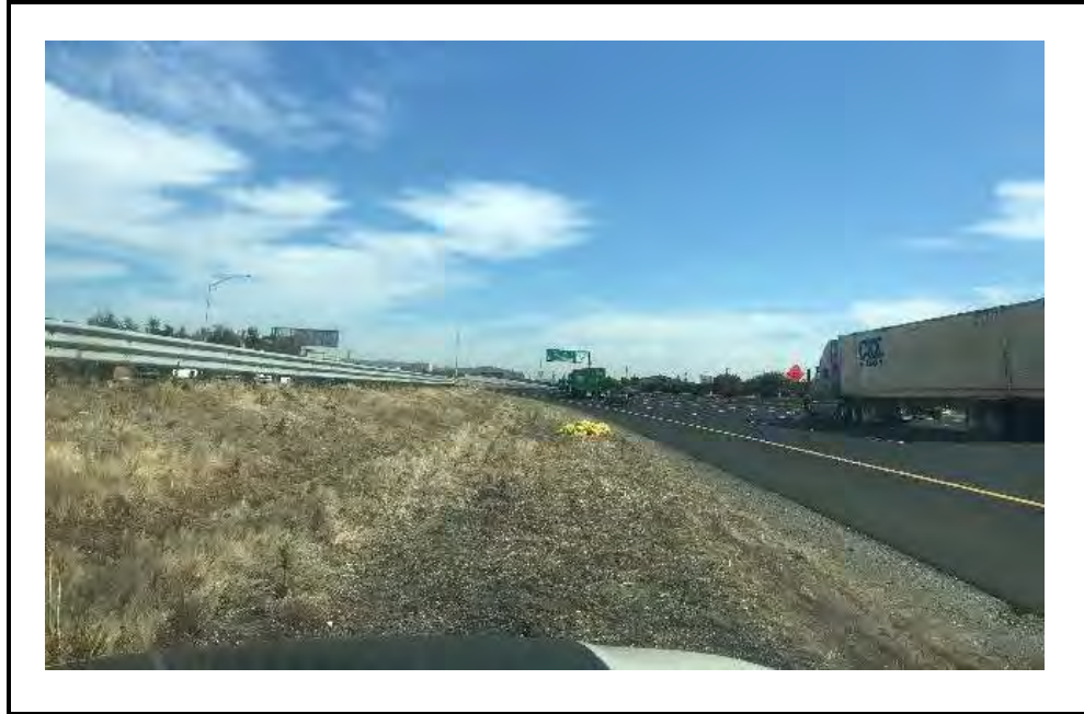
PHOTO C: VEGETATED STRIP AND SWALE - LOOKING UPSTREAM (NORTH EAST)
