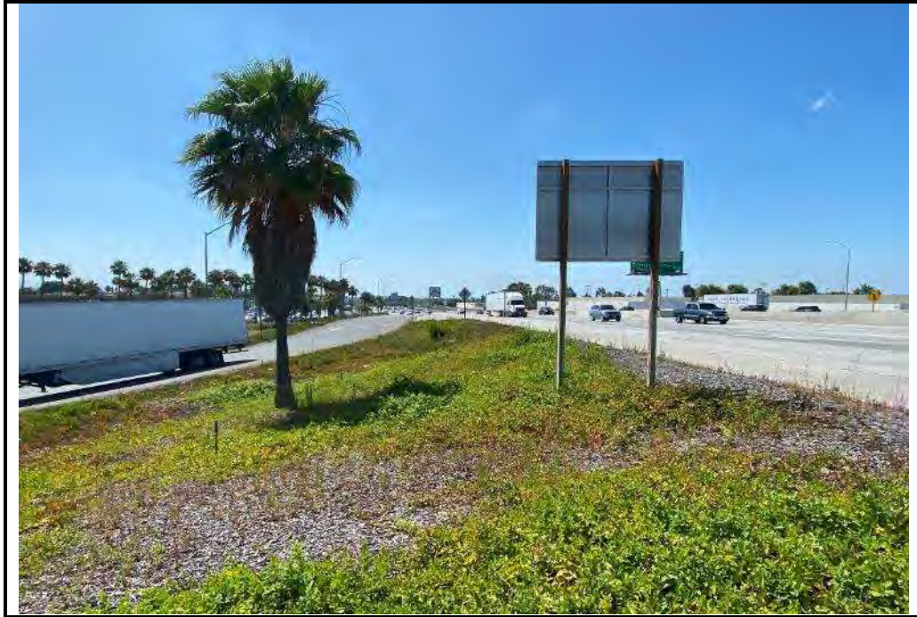
PHOTO C: Fill section with roadside vegetation strip slope between 2:1 and 4:1 (diked/curbed, 5-10' to ditch) (SOUTHEAST)
