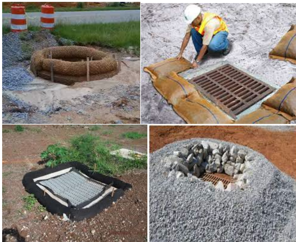
Figure 7: Engineering Controls at Field Inlets
