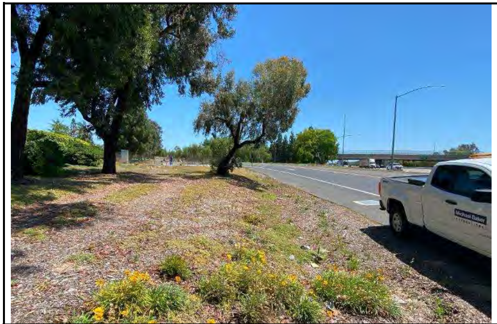
PHOTO B: Fill section with roadside vegetation strip slope flatter than 4:1 (sheet flow, 5'-10' to ditch) (SOUTH)
