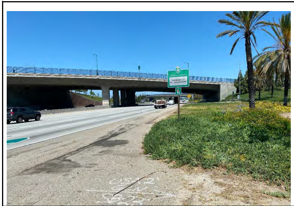
PHOTO B: Fill section with roadside vegetation strip slope flatter than 4:1 (diked/curbed, 10'-20" to ditch) (NORTHEAST)
