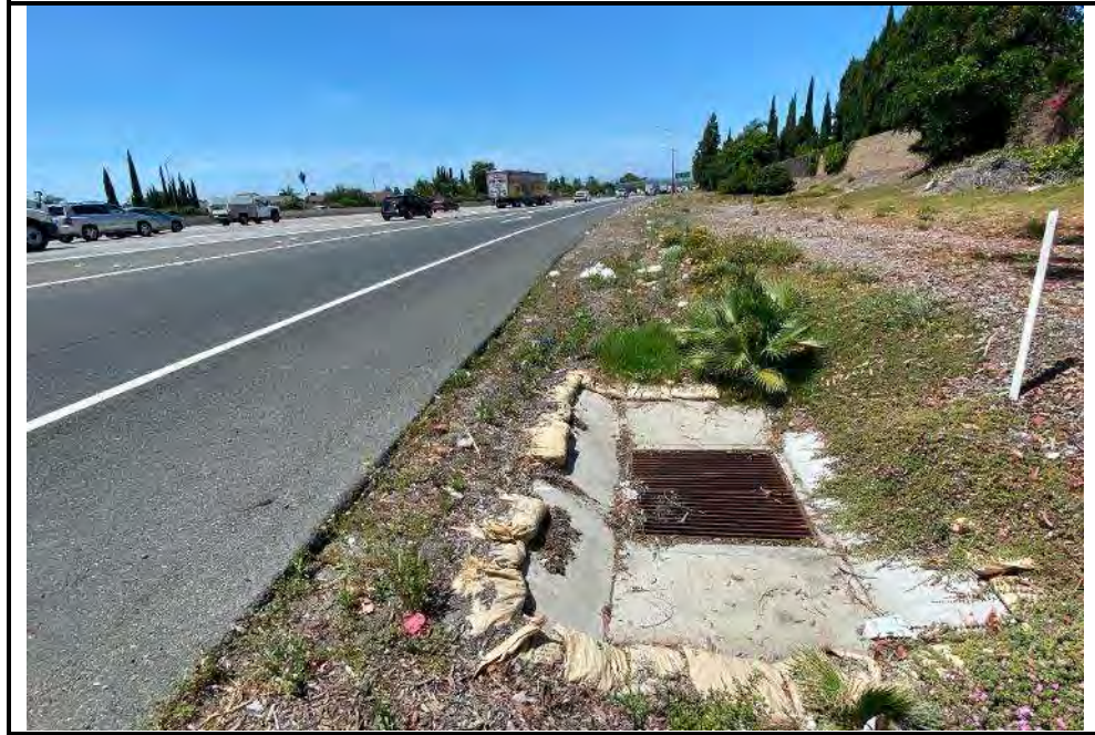
PHOTO A: Fill section with roadside vegetation strip slope flatter than 4:1 (sheet flow, 5'-10' to ditch) (NORTH)
