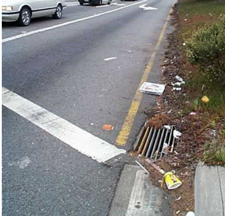
Common Inlet Grate
