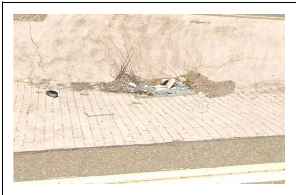
PHOTO B: CAPTURE DEVICE LOCATION TRASH AND DEBRIS OBSERVED AT GRATE
