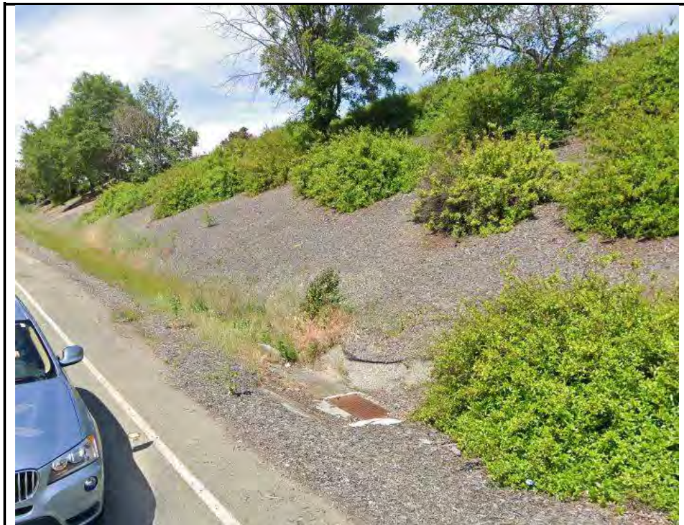
PHOTO D: VEGETATED STRIP AND SWALE AT DISCHARGE POINT (WEST)
