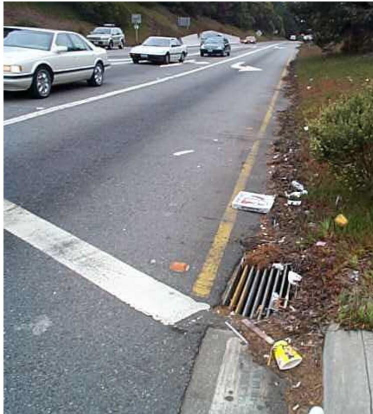
Common Inlet Grate
