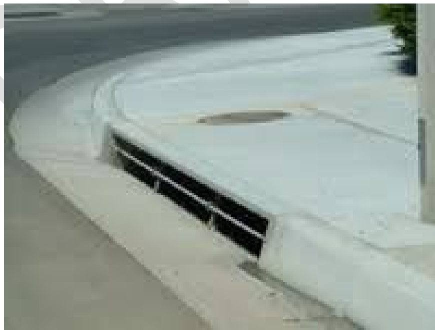
Less Common Curb Opening Inlet
