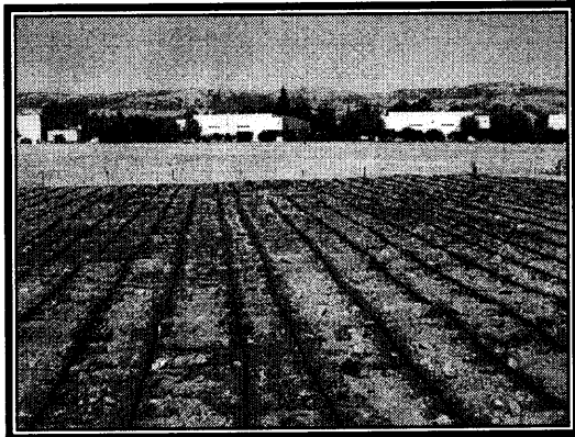
Photo 1 – This is a view, looking North, of the completed ex situ soil pile (sans cover). The drip tape is visible and the darker soil has been watered with perchlorate free site groundwater.
